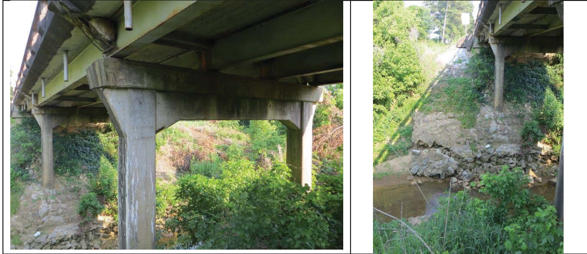
Figure 3. US 178 bridge with deep foundation- embankment eroded by scour (B-002)
