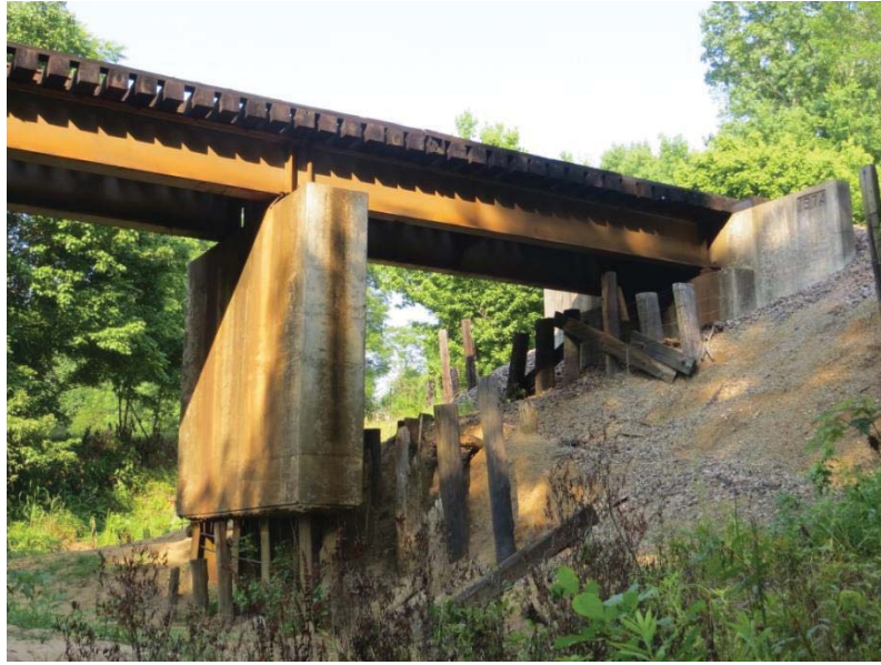
Figure 6. Railway bridge on deep foundation with piles exposed by scour.
