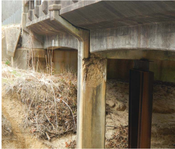
Figure 14. Bridge B-007 is located on the western edge of Sherman, Mississippi (lat. 34.451122, long. -88.760082) on Highway 178. Extensive damage to this bridge has required the insertion of an I-beam frame beneath the deck to assist in supporting the bridge. This bridge is considered a vulnerable to natural hazards such as earthquakes.
