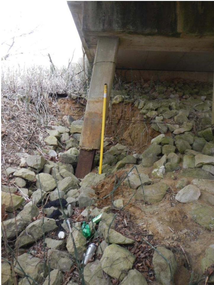
Figure 17. Above is an example of erosion originating from sources other than the stream channel. Downspouts direct the deck water downward forming linear gullying which expands to include the piers. Here (B-0013, lat. 34.44944, long. -88.83196 ) the gullying has exposed the piling to surface oxidation and erosion.
