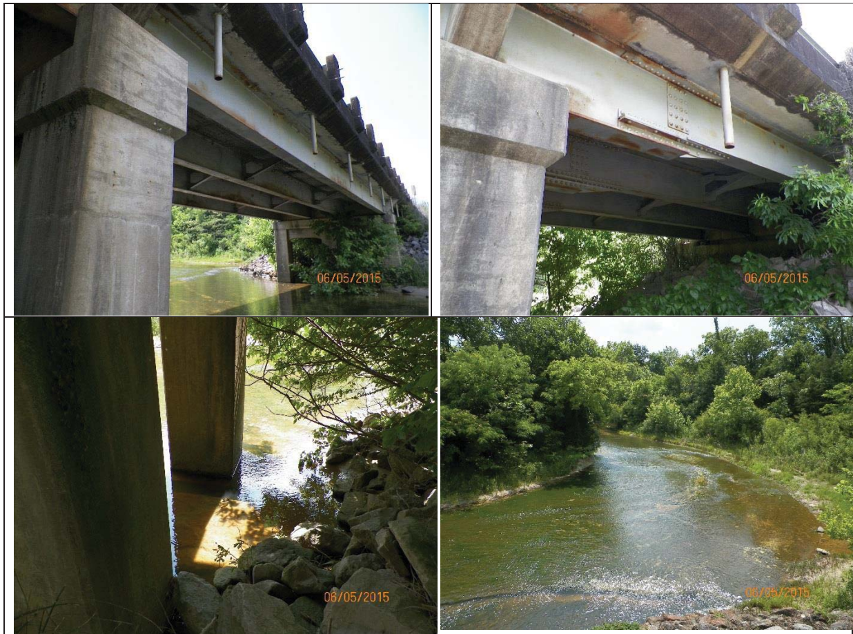
Figure 4. US 178 bridge with shallow foundation- footing exposed by scour (B-005)
