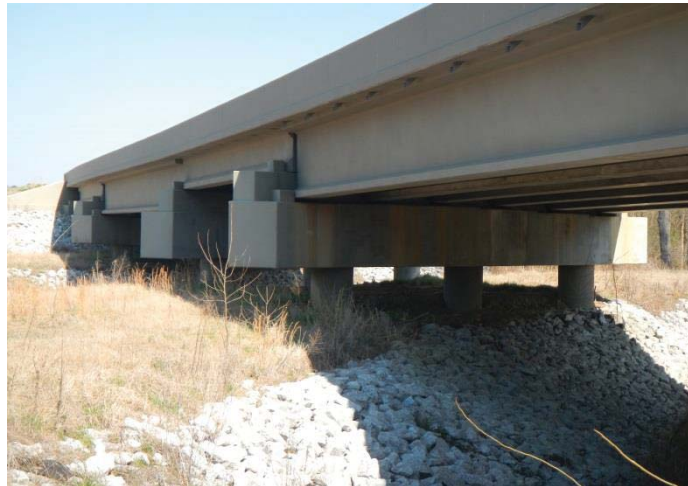
Figure 13. Bridge B-019 is a recent bridge on Mississippi Highway 9S in Pontotoc County. These new bridges are the least vulnerable within the study area. This bridge is approximately 0.8 mile from Endville, Miss. (lat. 34.311967, long.-88.888418). Neither this bridge nor any of the other bridges on the new portion of Highway 9 appear on the NBD.
