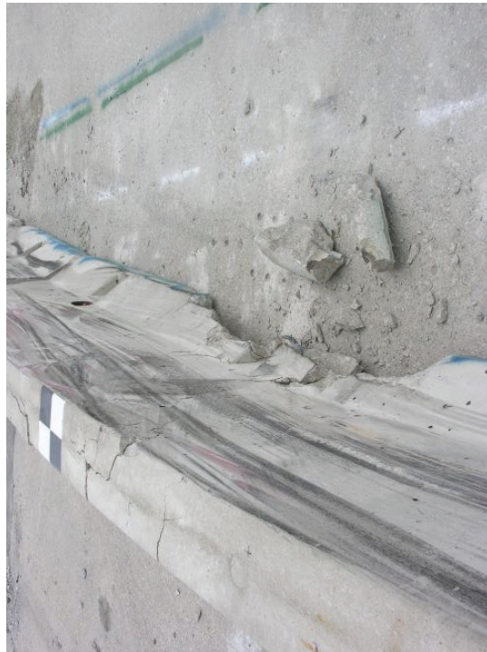
Figure 35. System Damage - Barrier No. 2, Test No. TTCB-1
