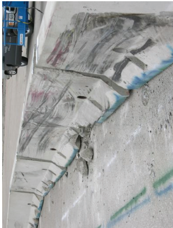
Figure 33. System Damage, Test No. TTCB-1
