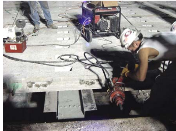
Figure 13: Post tensioning sections together. (Note: only one of two rods being tensioned to 90,000 lbs. at same time is shown)
