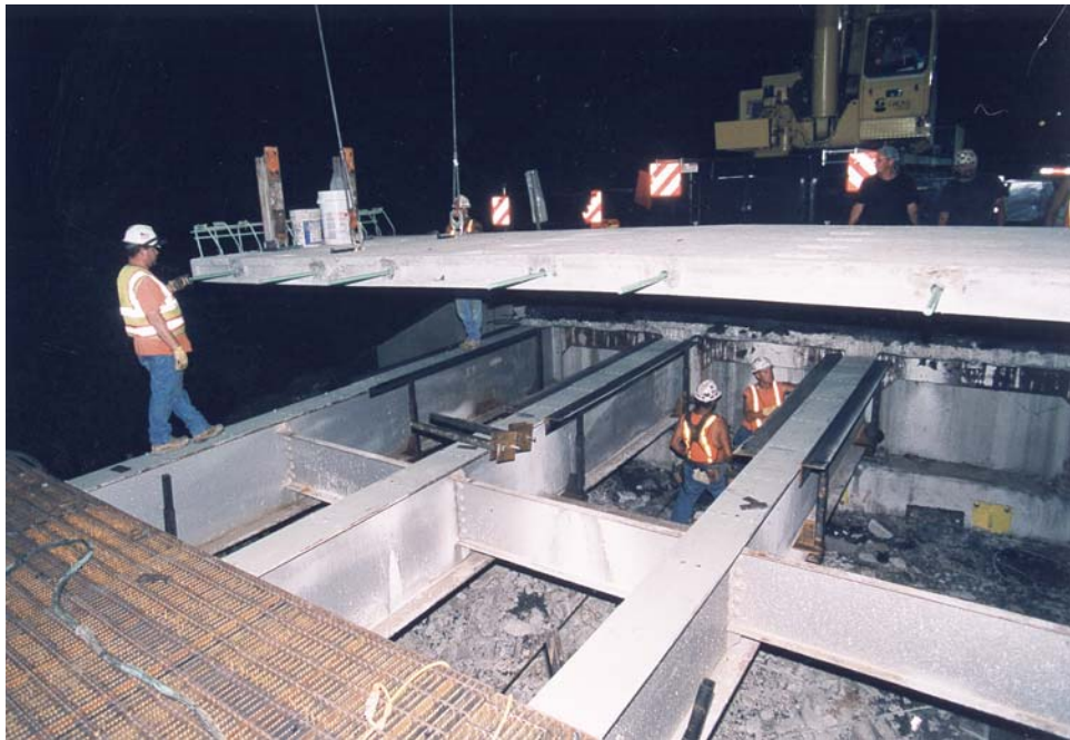
Figure 11: Setting the first precast panel, Note: Workers under bridge are adjusting jacks for the haunch forms to match the crown cast into the bottom of the deck and bring to proper grade before filled with fast setting grout. Note: Temporary steel deck panel in place in foreground.
