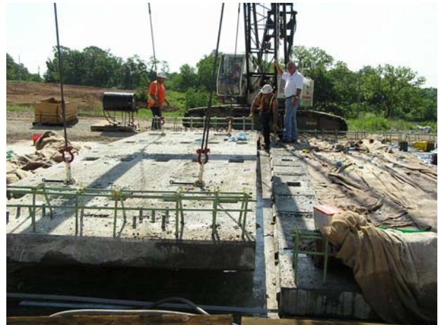
Figure 6: Lifting completed panel from casting bed. Note: keyways showing on edge of opposite panel.
