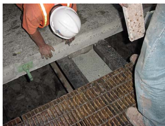
Figure 15: Removing 2x4 used to form end of haunch after grout set in about 2 hours.
