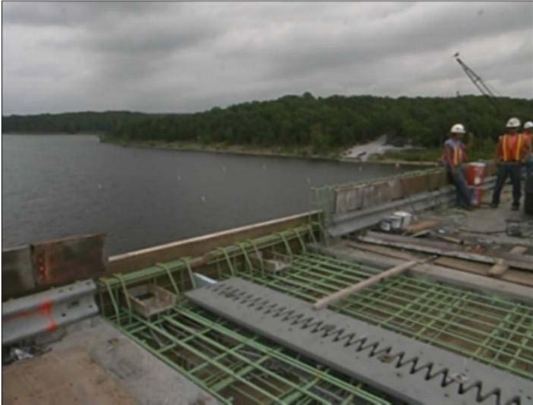
Figure 16: getting ready for placement of concrete between precast sections and around new finger expansion joint.
