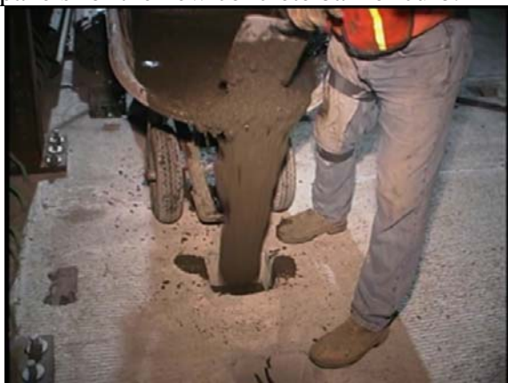
Figure 14: Pouring grout into 2nd of 4 blockout holes per girder line in precast panel.
