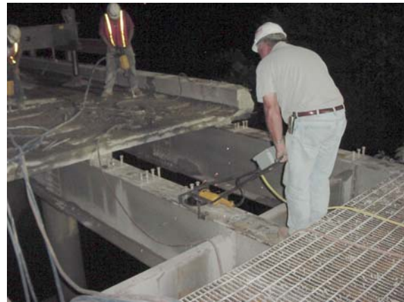
Figure 8: Background – Jackhammering around shear studs to loosen old deck Foreground – Sawing off steel shear studs after old concrete deck removed.
