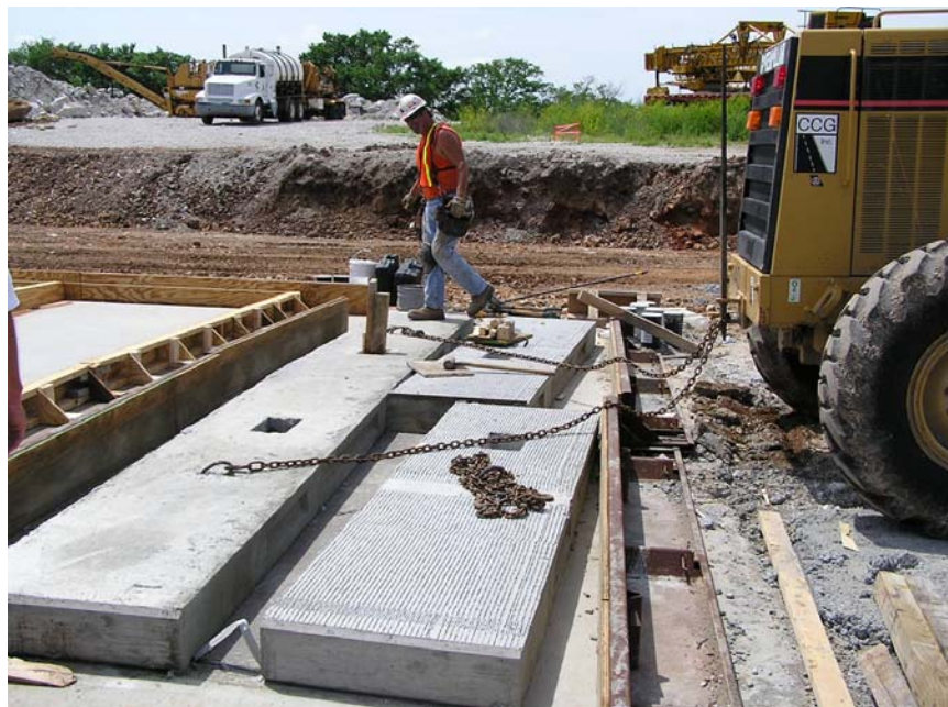
Figure 3: Trial match-cast sections showing keyways on both sides of panels. One side against forms and one side against concrete.
