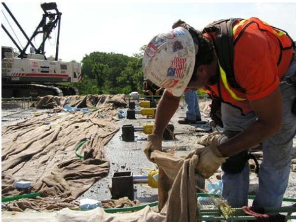
Figure 5: Jacking match-cast panels apart using square steel posts set in blockouts on each side of joint with release agent applied to it
