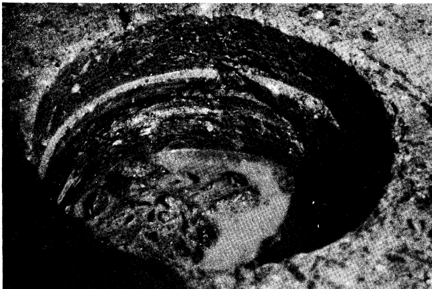
Figure 19. Cross section view of the delaminated spot showing extremely wide separation of concrete layers.
