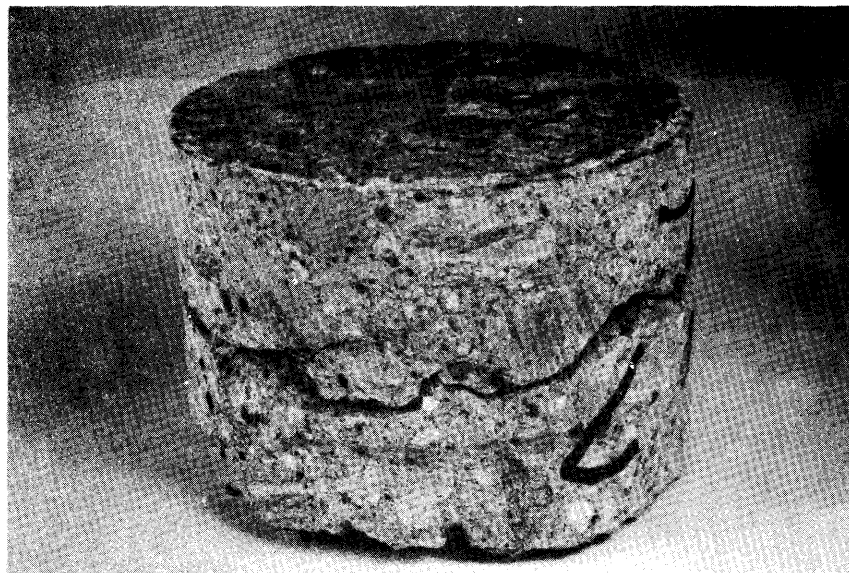
Figure 25. A core from a delaminated spot in square 2-7 in Figure 13.
