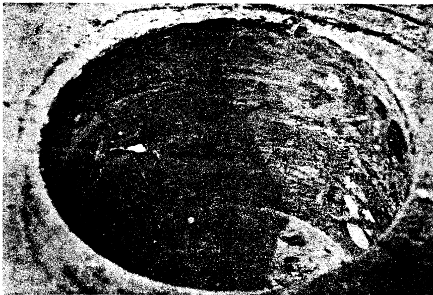
Figure 21. A cross-section view of the delaminated spot. Notice that the separation between concrete layers is narrower than that shown in Figure 19.
