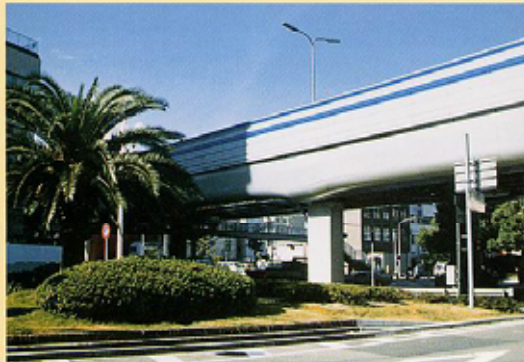
Photo 2 The noise barrier uses aluminum decorated plates to emphasize the horizontal line and to hide the pillars, and the beam side is covered with the panel having similar features, thereby ensuring fine views.(Kobe Line,Hanshin Expressway NO.3)
