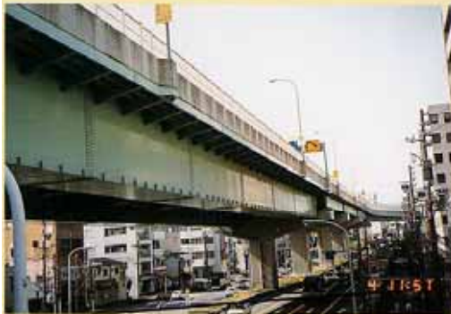
Photo 9 Installation of the translucent plate sound barrier protects sunshine and landscape. (Nagoya Expressway Branch NO.3)
