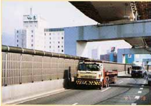
Photo 7 Installation of the noise reducer (cylindrical noise absorber on the top of the noise barrier) reduces diffraction noise, giving a greater effect than expected from the barrier height. This is effective when the barrier height is restricted. (Hamanote Bypass, National Highway NO.2)
