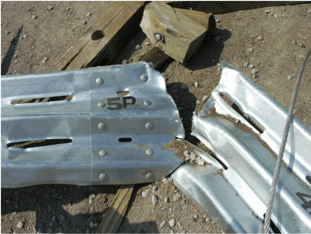
Figure 93. Rail Tear, Test SR-8
