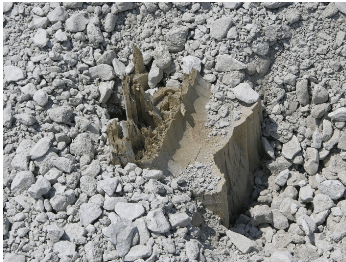
Figure 52. Post Nos. 3S through 5S Damage, Test SR-7
