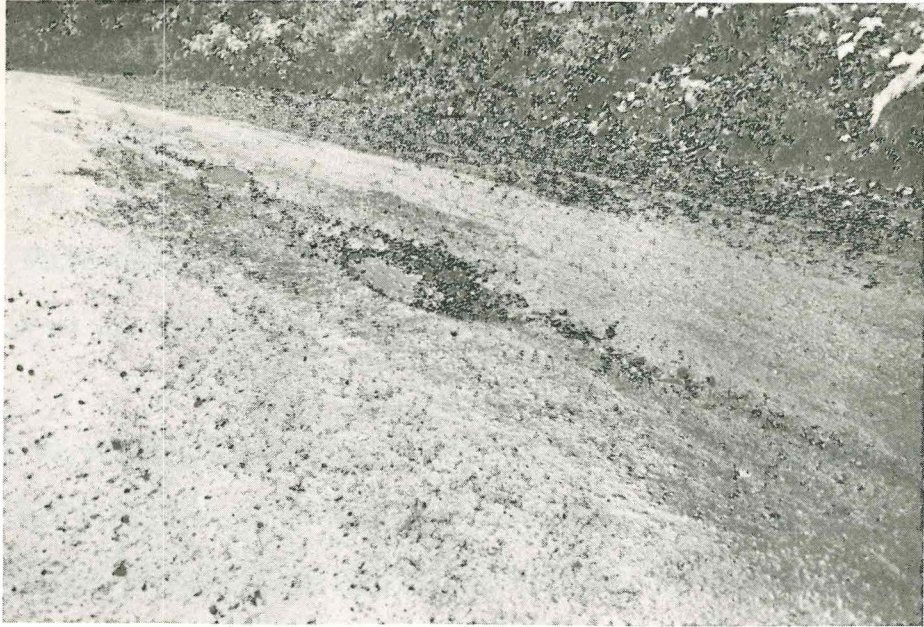
Figure 8. Nestucca Access Road below McMinnville reservoir. Water-filled breaks in paving showing base aggregate failure. October, 1973.
