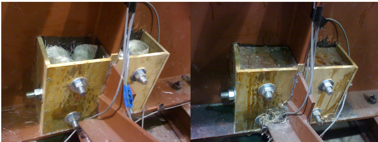
Figure 3: GFRP Repair Block for Girder Subassembly 1 Prior to Casting the West System™ Resin and After Curing
