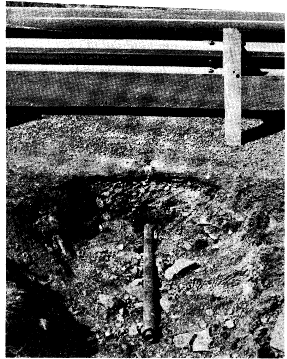
Figure 15. Equipment used to bore under the road and an installed pipe sleeve.
