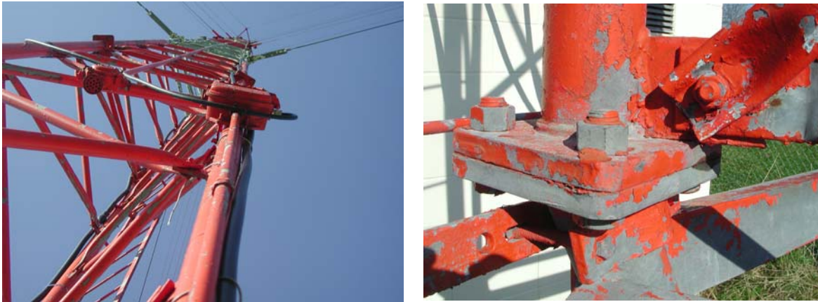
Figure 2.12. Details of Ashland central mast. Significant paint flaking is observed but minimal loss of galvanization.
