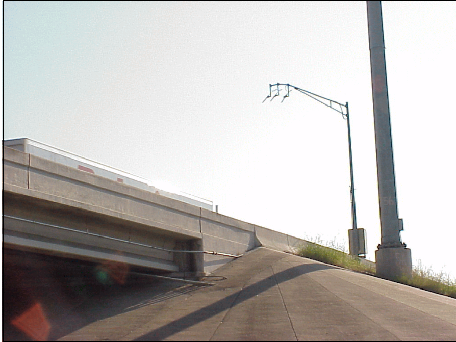
FIGURE 3-12 US 290 at the Second AVI Antenna Taken Looking Up from Gessner
