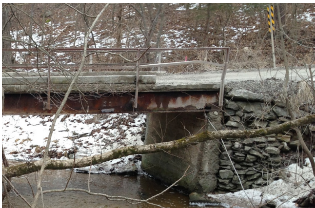
Original Rustic Road bridge showing deterioration of the outer girder, including corrosion through an entire portion of the web near the abutment
