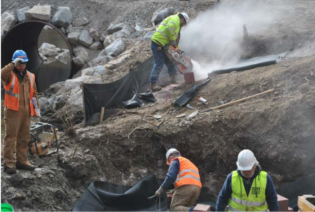
Figure 16. Concrete saw being used to cut CMU block for corner of north abutment
