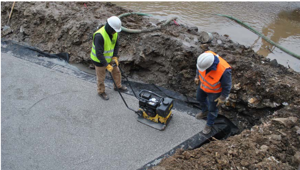
Figure 11. Compaction of second course for south abutment with worker standing on corner blocks to prevent movement
