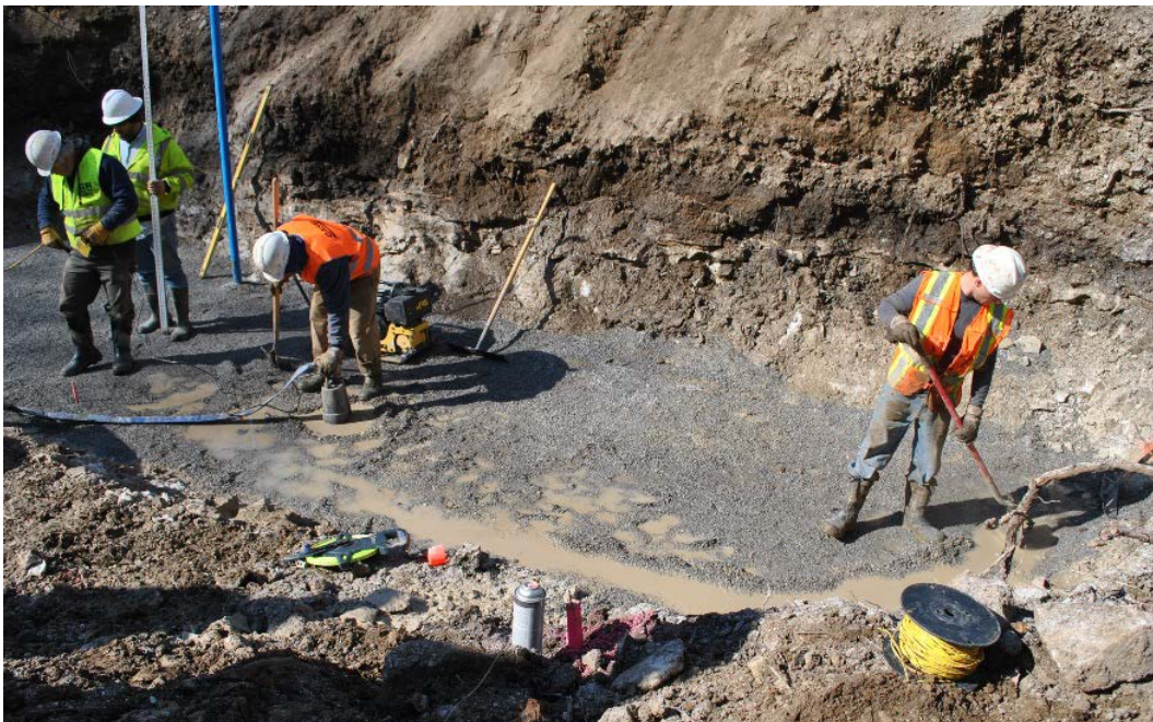
Figure 15. Pump being used to remove seepage water from north abutment prior to compacting
