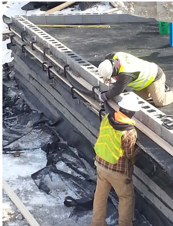
Figure 21. Securing boards to reinforcement to prevent movement of the CMU blocks during compaction
