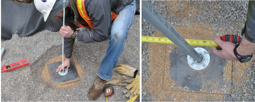
Figure 36. Installation of bottom settlement plate: placement and leveling on thin layer of coarse sand (left) and placement of loose PVC sleeve over steel rod to prevents friction between rod and aggregate (right)
