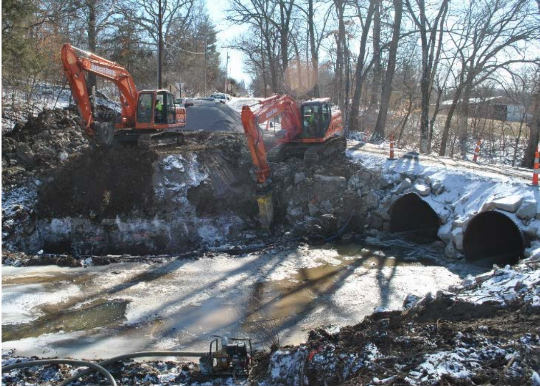
Figure 8. Rock chipping hammer and backhoe being used to excavate limestone bedrock below south abutment
