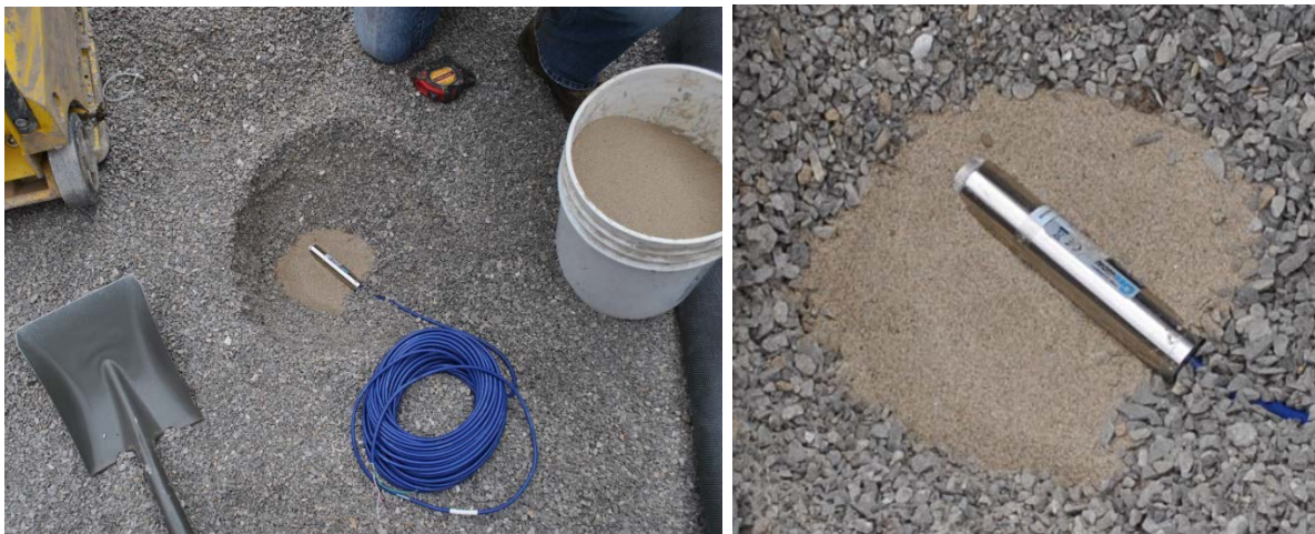
Figure 40: Piezometer PZ-1: installation in sand pocket within GRS backfill (left) and close-up view of vibrating wire piezometer (right)
