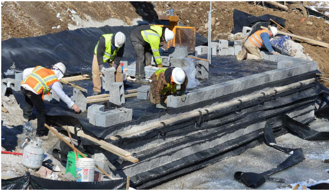
Figure 20. Leveling CMU blocks ahead of placing backfill with boards clamped to reinforcement used to prevent movement of blocks for previous course during compaction
