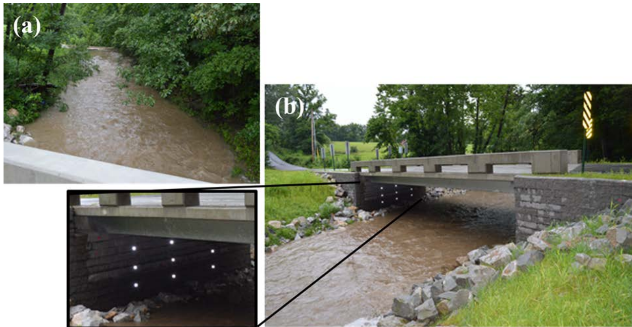
Figure 41. Rustic Road GRS-IBS during July 2015 high water event: looking upstream from on top the bridge showing creek high up its banks (upper left) and looking at north abutment (right) with close-up view (lower left)
