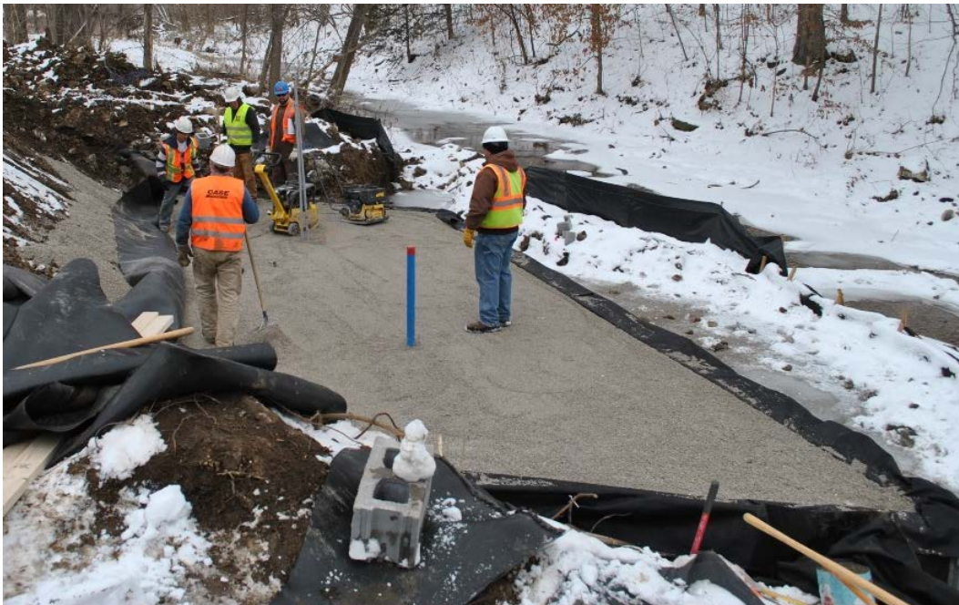
Figure 17. Compacting tenth course of GRS of north abutment after placing second telltale device for measuring settlement
