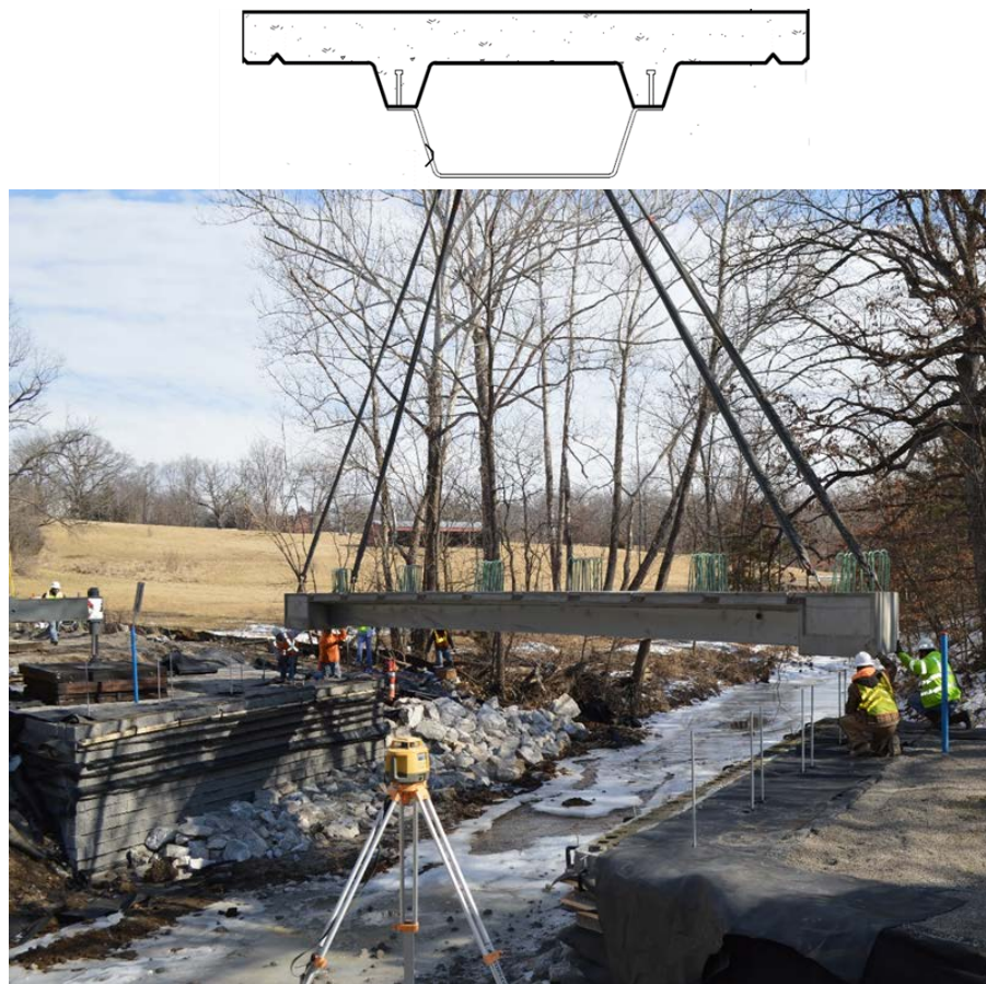
Figure 6. Tub girders with precast bridge deck: cross-section (top) and tub girder being lowered into place (bottom)
