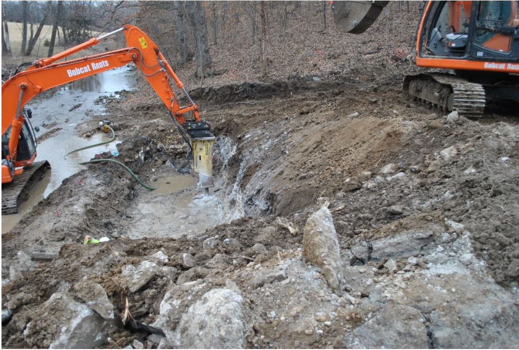
Figure 7. Rock chipping hammer being used to excavate limestone bedrock below south abutment
