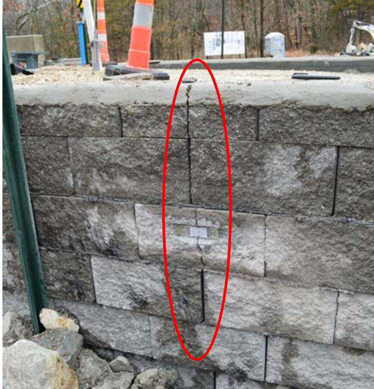
Figure 43. Crack on east wing of north abutment wall
