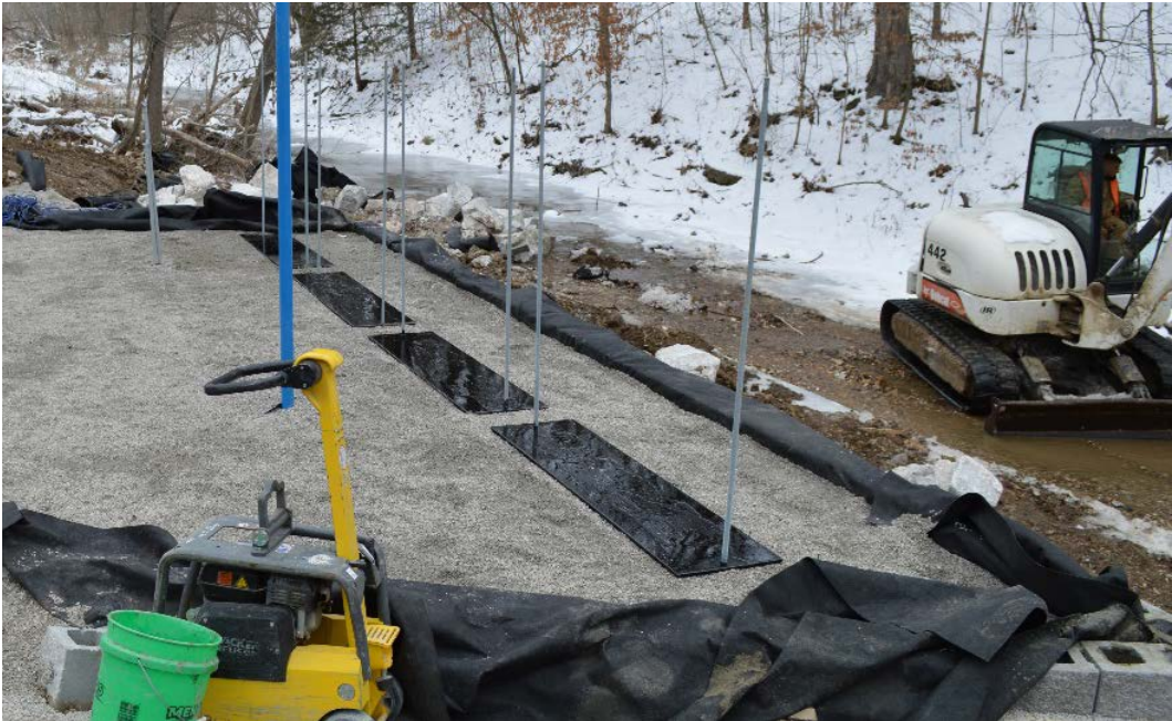
Figure 23. Four anchor plates (one per girder) placed approximately 3 ft below the top of each abutment within the backfill
