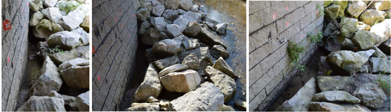
Figure 42: Downstream corner of south abutment: August 31, 2015 (left), February 25, 2016 (center), and September 22, 2016 (right)
