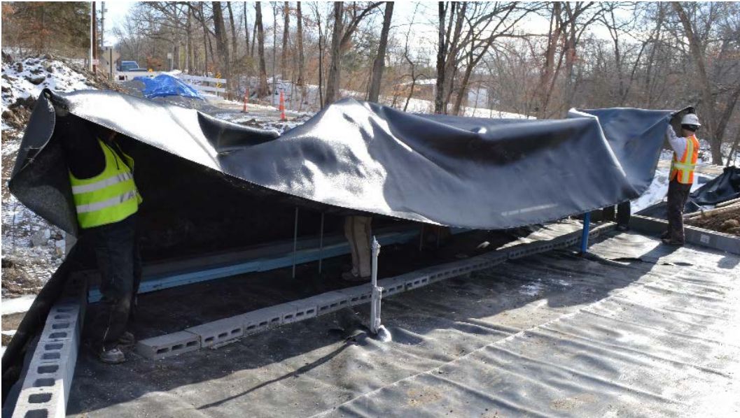
Figure 25. Placement of reinforcement for bottom layer of beam seat for north abutment
