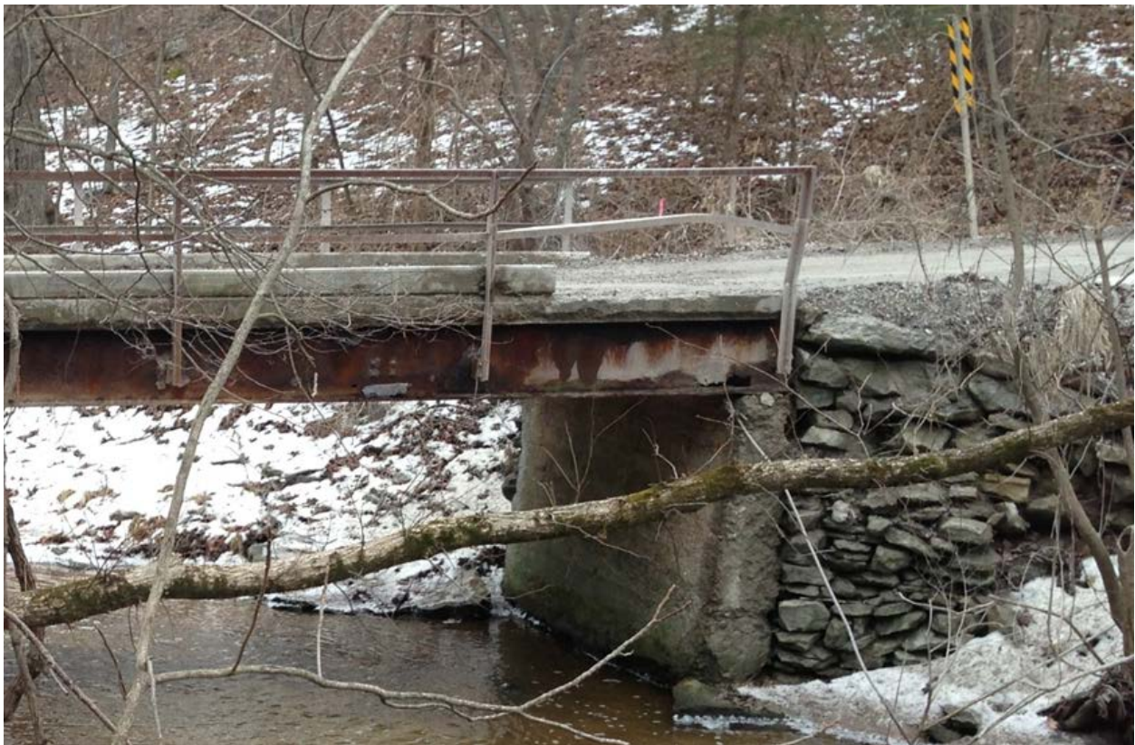
Figure 5. Original Rustic Road bridge showing deterioration of the outer girder, including corrosion through an entire portion of the web near the abutment
