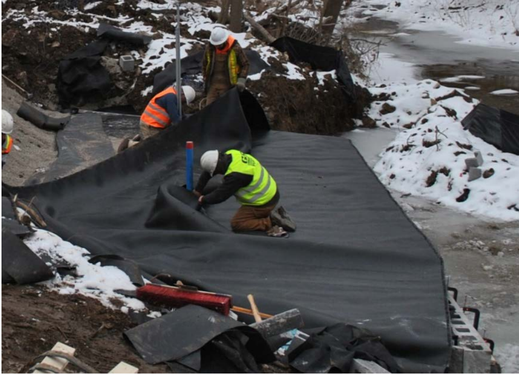
Figure 18. Placing reinforcement around instrumentation (inclinometer and telltales) atop tenth course of GRS of north abutment
