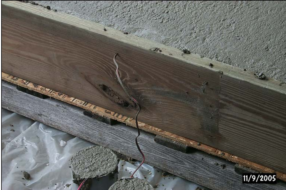
FIGURE B11 Maturity meter wire protruding out side of test slab.
