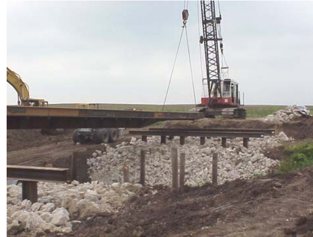
b. Placement of the 89-ft RRFCs
