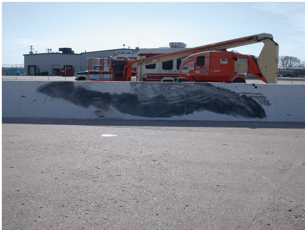
Figure 35. System Damage, Test No. ZOI-1
