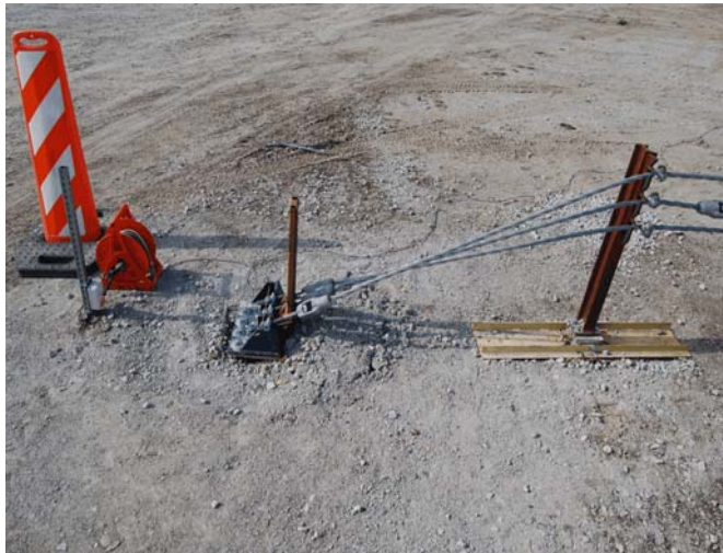
Figure 34. End Anchor Damage, Test CS-2
