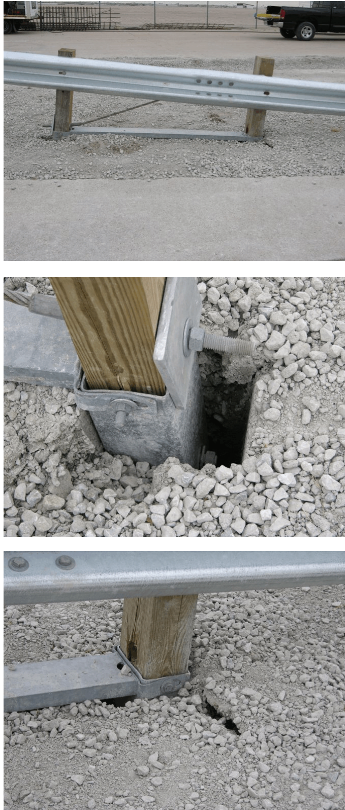
Figure 63. Upstream Anchorage Damage, Test No. MGS221-2
