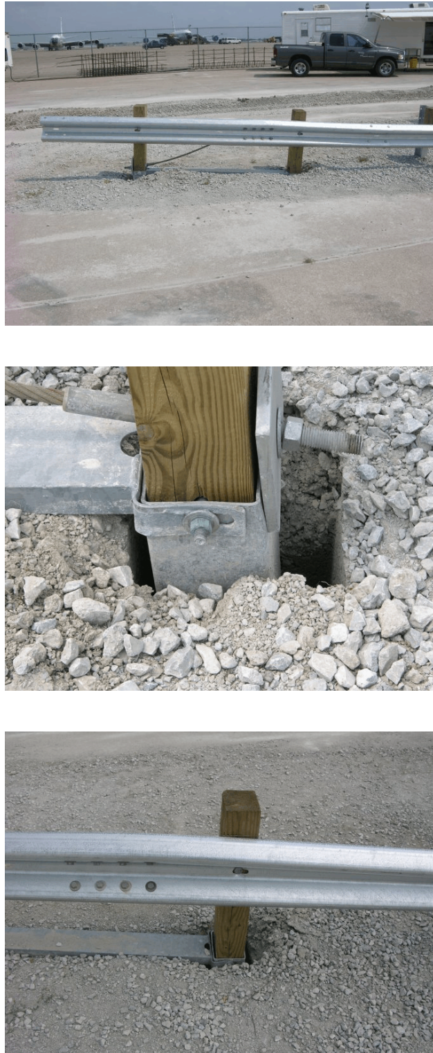
Figure 40. Upstream Anchorage Damage, Test No. MGS221-1
