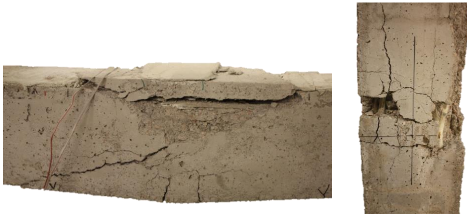
Figure 4.29 Surface constrictive cracking in IIa-1 (left: side view, right: bottom view)
