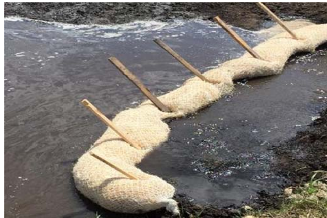
Figure 4.2 Undercutting observed underneath the product.
