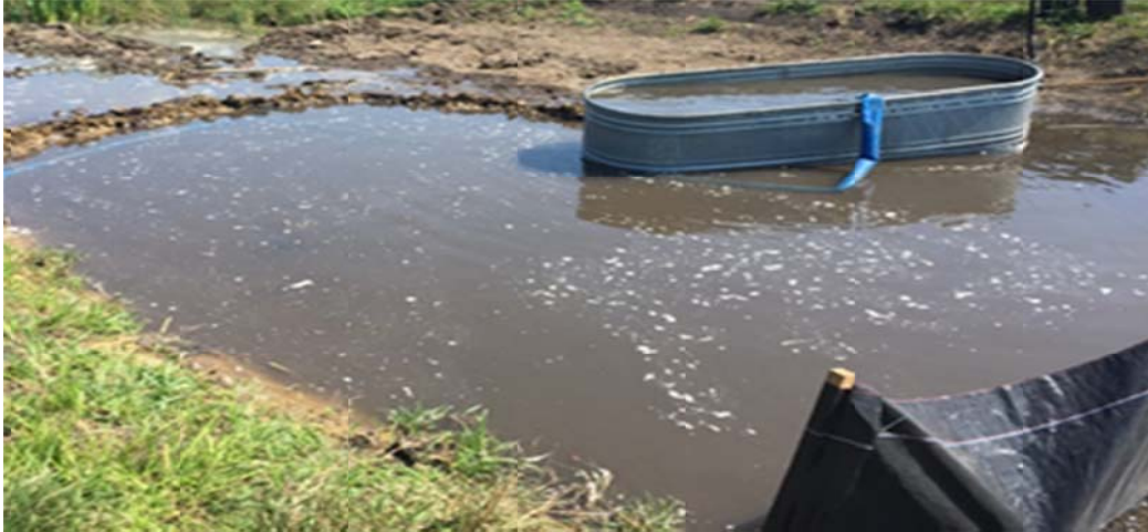
Figure 4.8 Heavy ponding (silt fence with IDOT-approved fabric).
