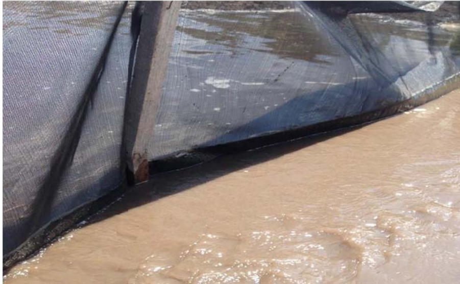
Figure 4.6 Observed water level difference upstream and downstream of the silt fence (woven monofilament).
