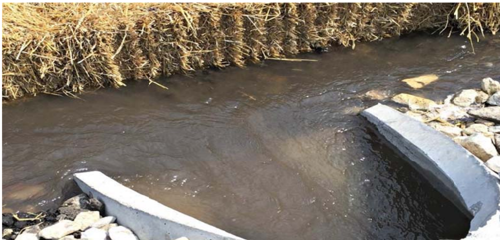
Figure 4.15 Unfiltered sediment entering inlet.
