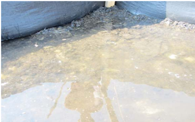
Figure 4.17 Undercutting of silt fence.
