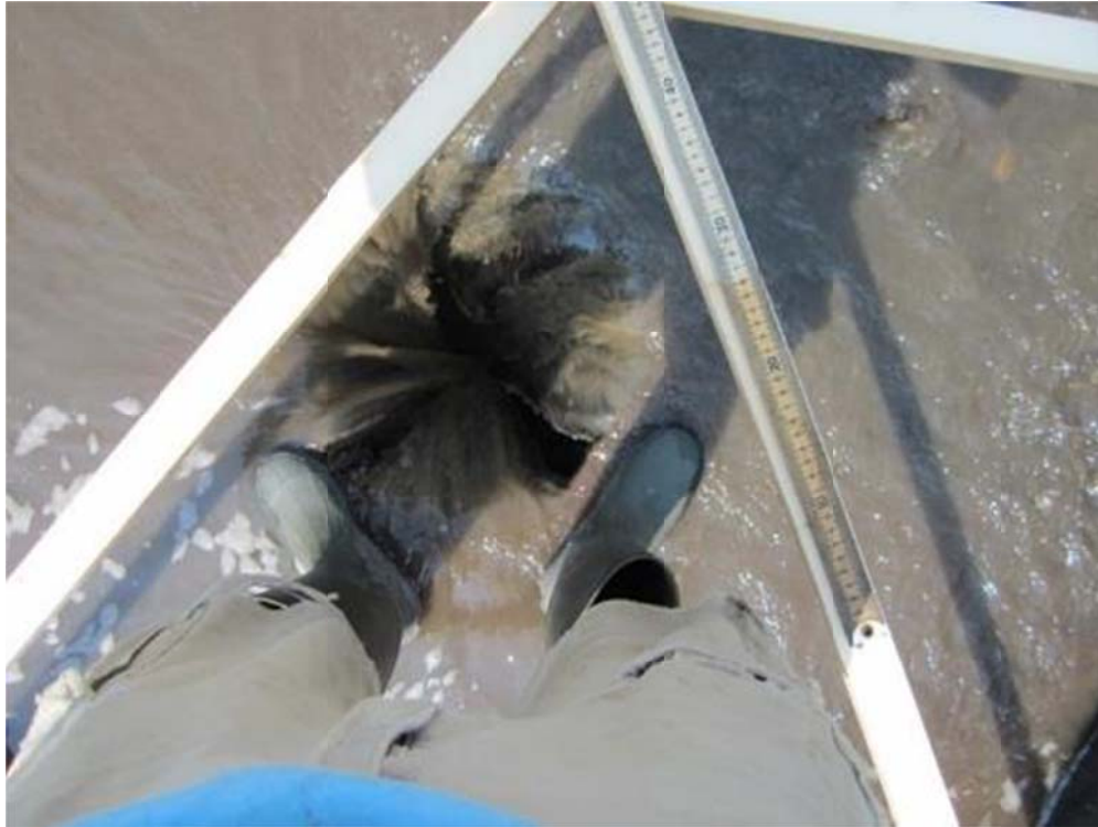
Figure A.19 Silt fence (2 foot gap) product failure.
