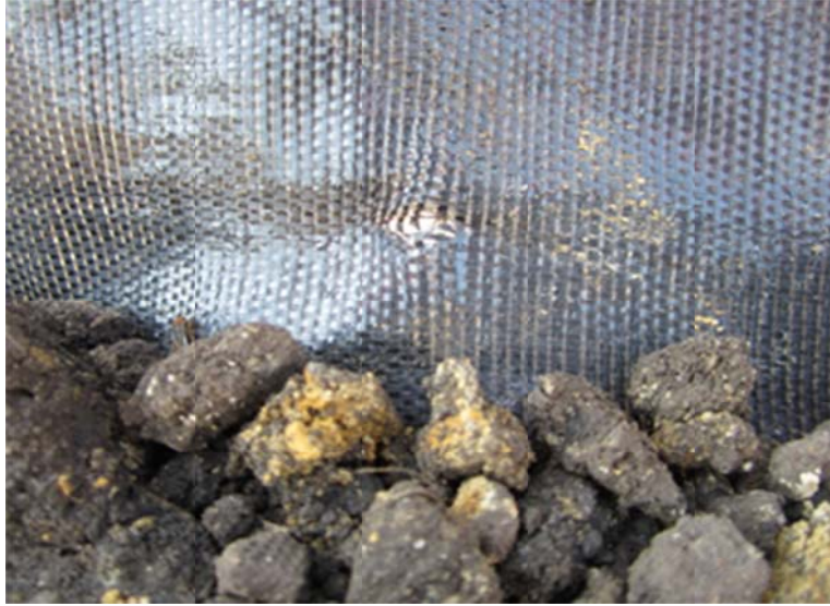
Figure 4.16 Tear in silt fence.
