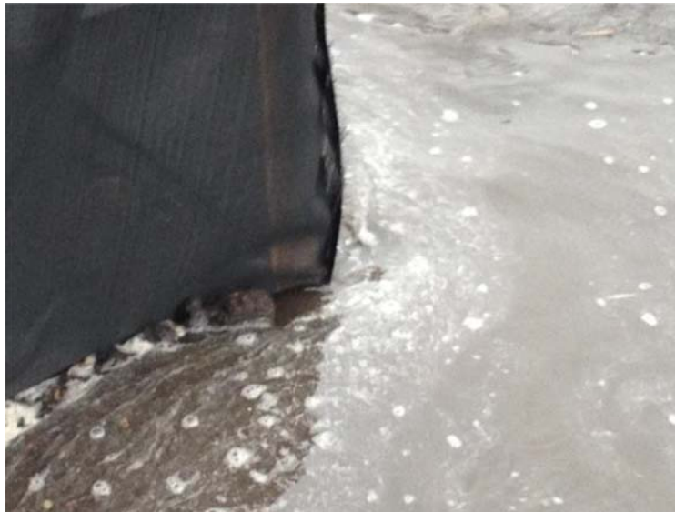
Figure 4.19 Rapid flow around the side of the silt fence (monofilament fabric).
