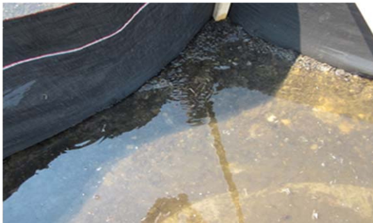
Figure 4.18 More undercutting of silt fence.
