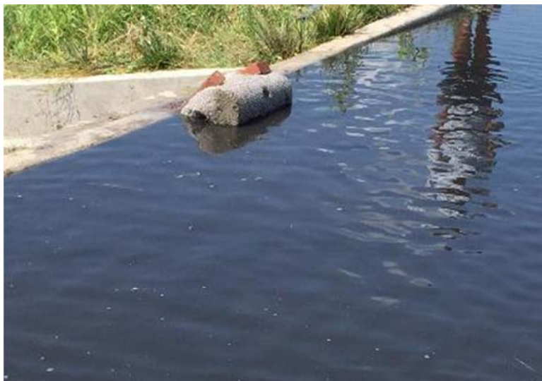
Figure 4.11 Water overtopping curb (GeoHay).
