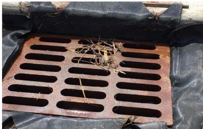
Figure 4.23 Exterior debris after draining slab (Inlet Pro).
