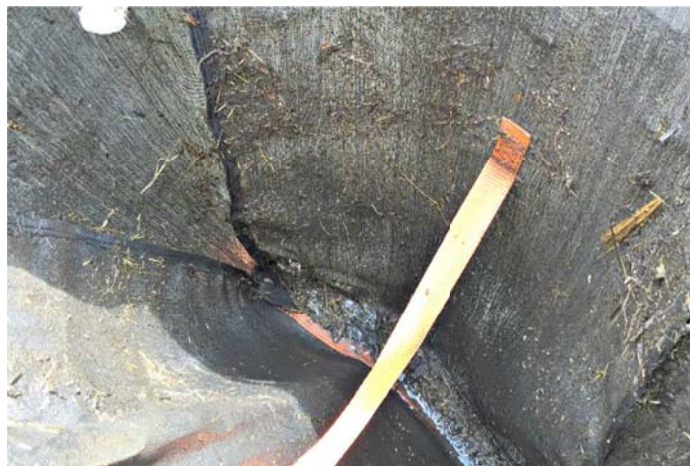
Figure 4.24 Accumulated sack residue after draining slab (Inlet Pro).
