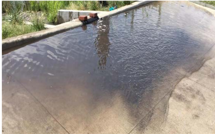
Figure 4.20 Inlet Pro accumulated ponding.
