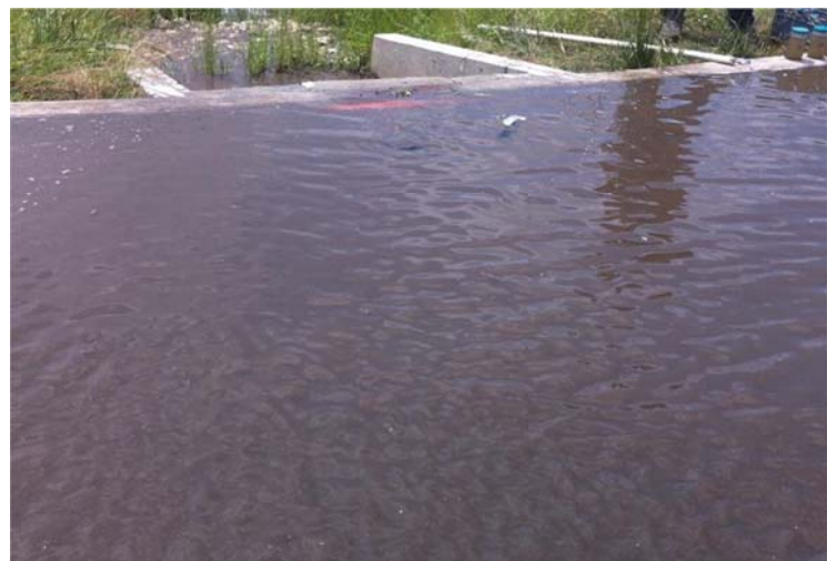
Figure 4.9 Water overtopping curb, product failure (Dandy curb bag).
