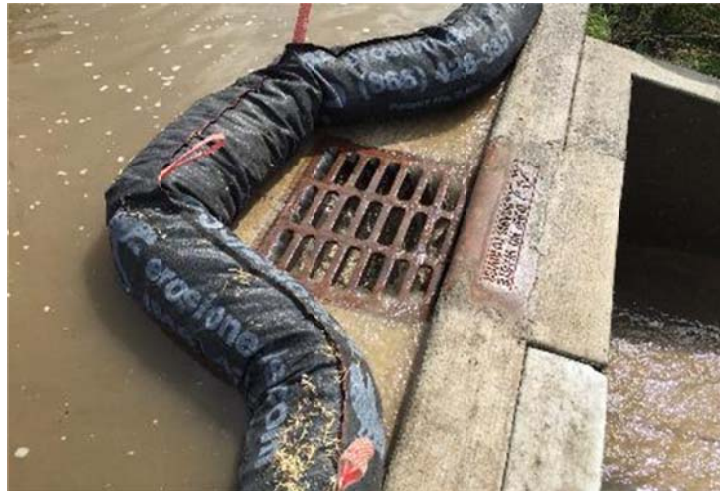
Figure 4.13 Erosion Eel draining.
