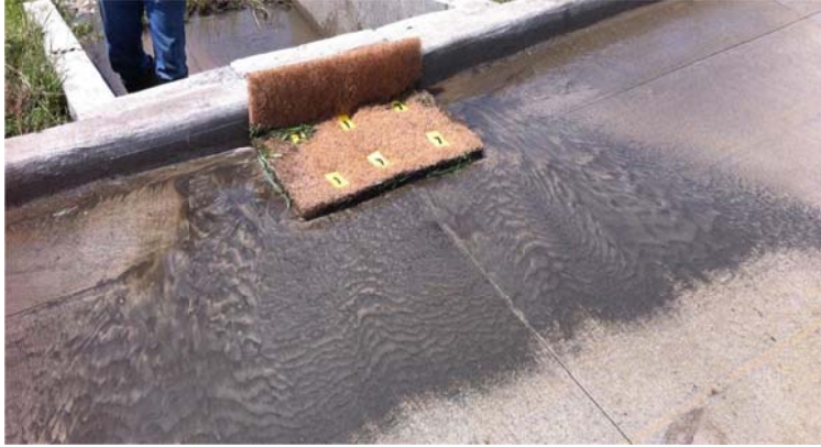
Figure 4.17 Sediment residue around SediGuard after slab was drained.
