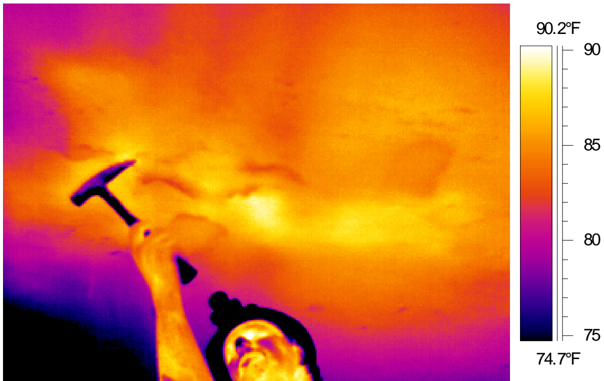
Figure 39 – Thermal image of Heating Location # 1: excavating a detected flaw
