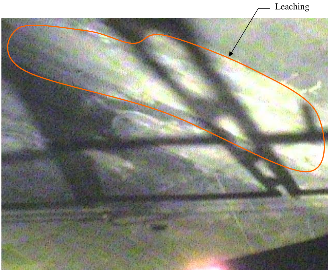
Figure 35 – Photo of Heating Location # 1 with extensive discoloration due to leaching
