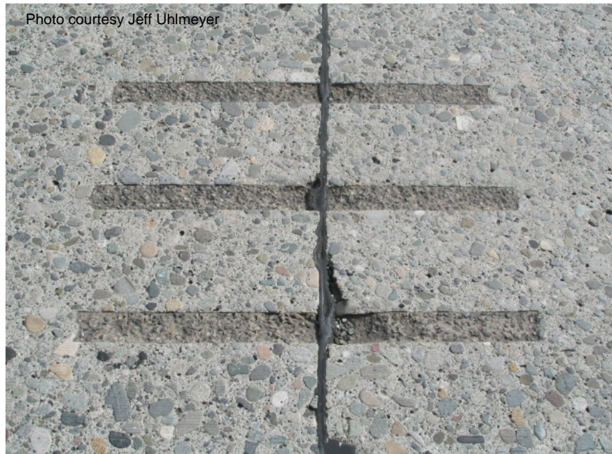
Figure 45 Spalling of patching material.
