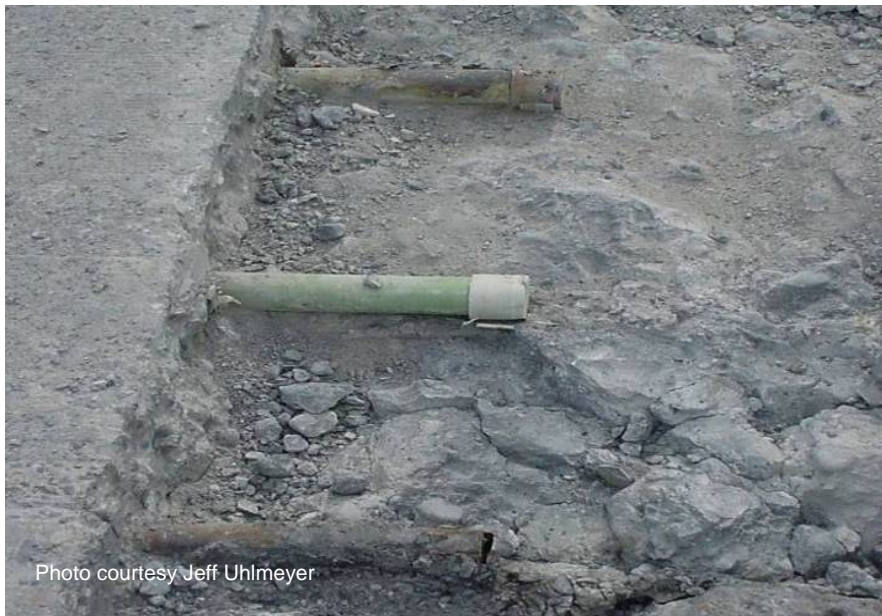
Figure 59 Close-up of corroded epoxy coated dowel bars.
