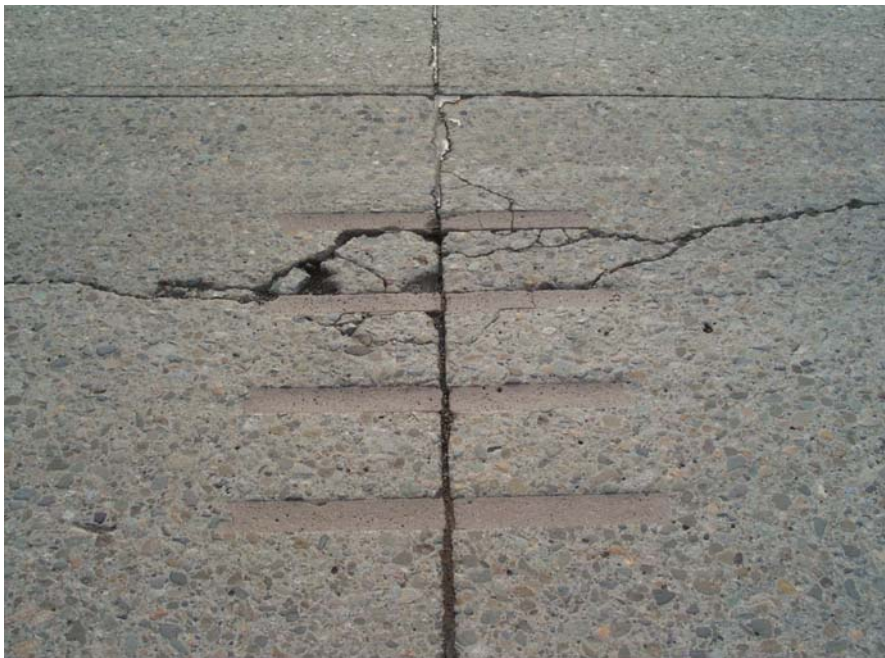
Figure 20 Severe failure of dowel bar slot placed over existing longitudinal crack.
