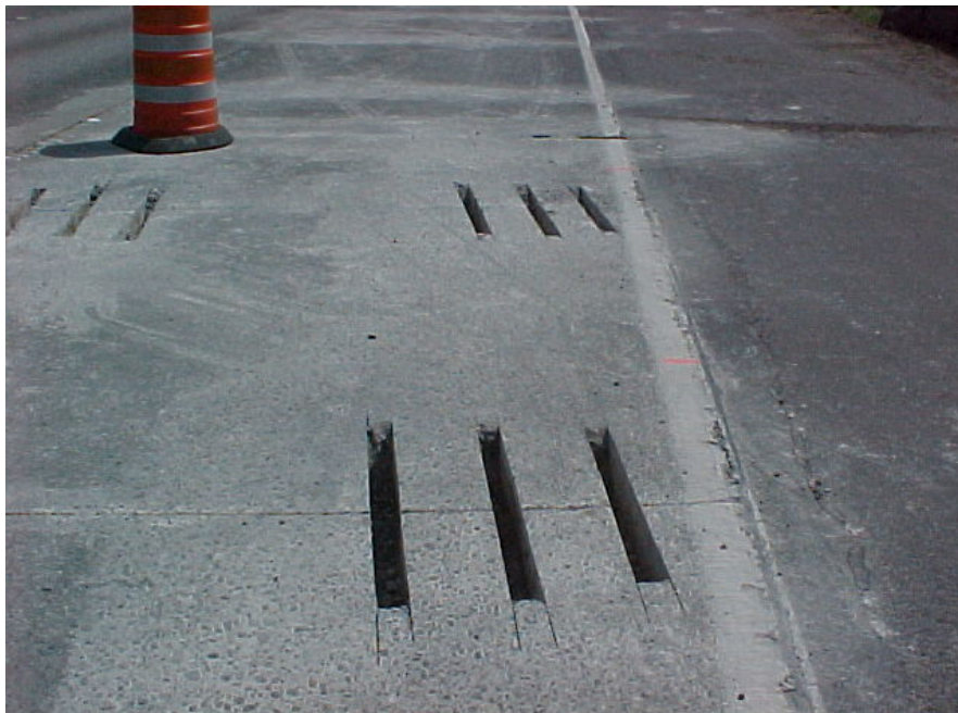
Figure 14 Dowel bar slots incorrectly cut on skewed joints.
