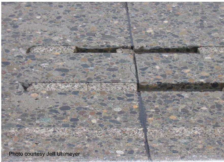
Figure 44 Severe patching material bond failure.
