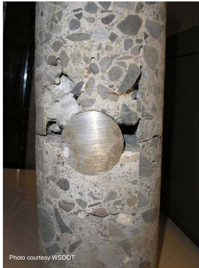
Figure 69 Poor consolidation around bar.
