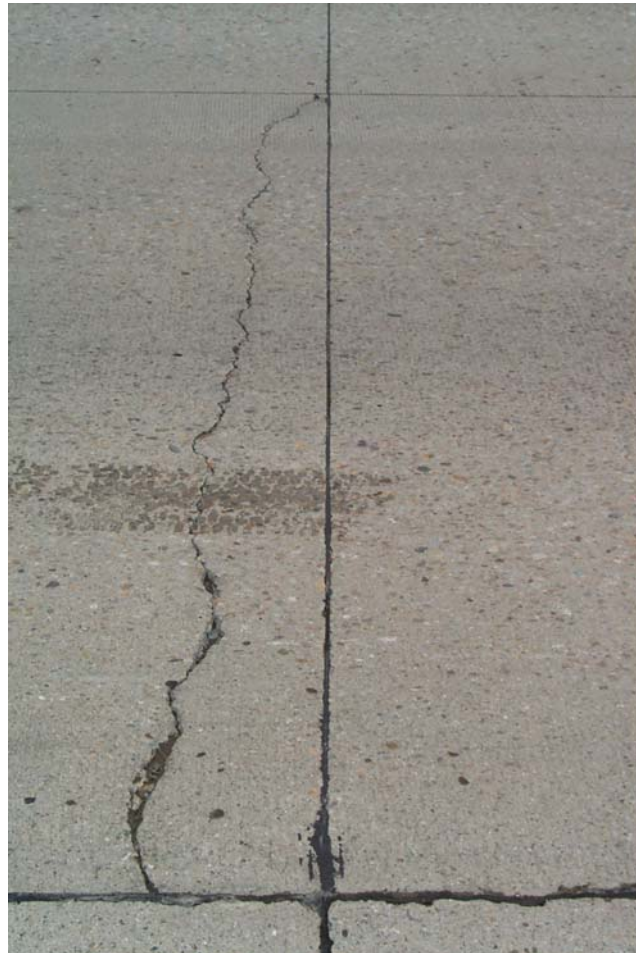
Figure 21 Transverse crack is functioning as the working joint.
