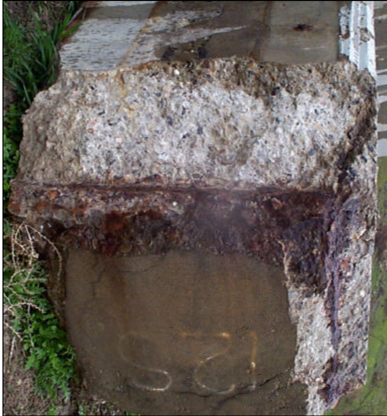
Figure 1.5 – Bent 12S, deterioration at tip of cantilever
