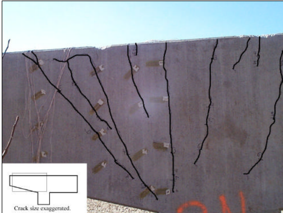
Figure 5.51 – Bent 2N, cracks on cycle 7.
