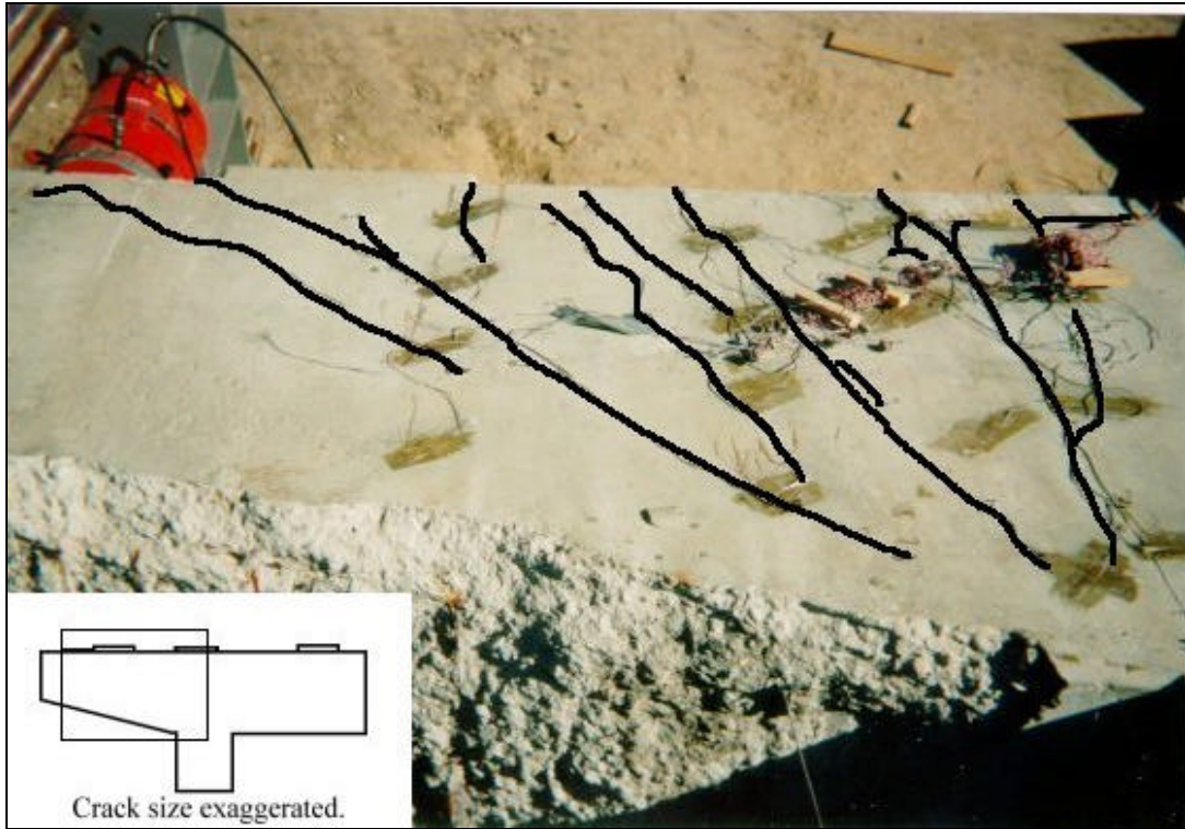
Figure 5.16 – Bent 12S, cracks on cycle 8.
