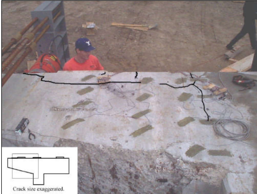
Figure 5.25 – Bent 12N, cracks on cycle 5.
