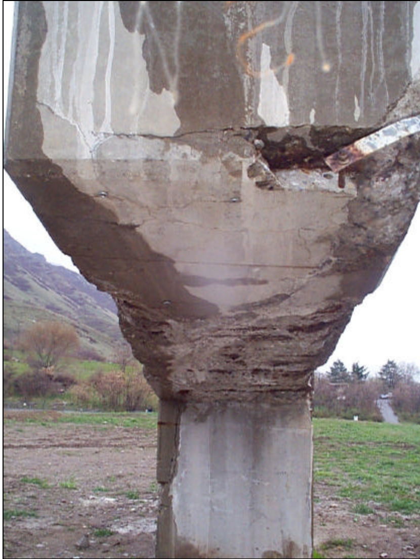
Figure 1.7 – Bent 12N, deterioration on underside of cantilever
