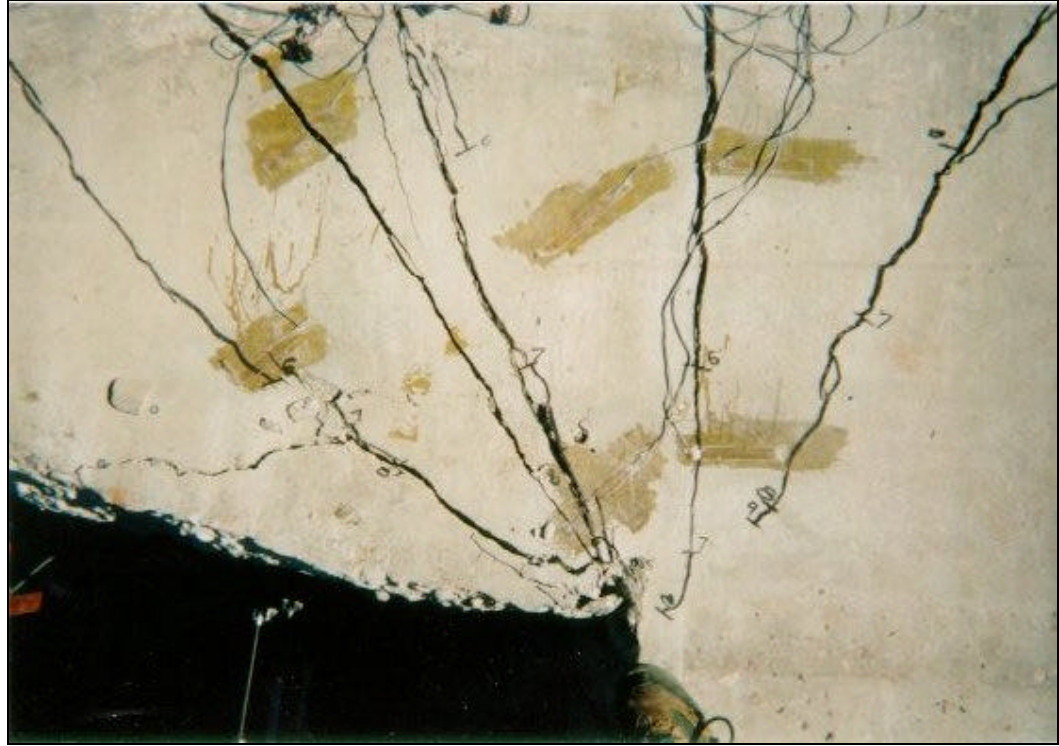
Figure 5.20 – Bent 12S, Compression zone after failure.
