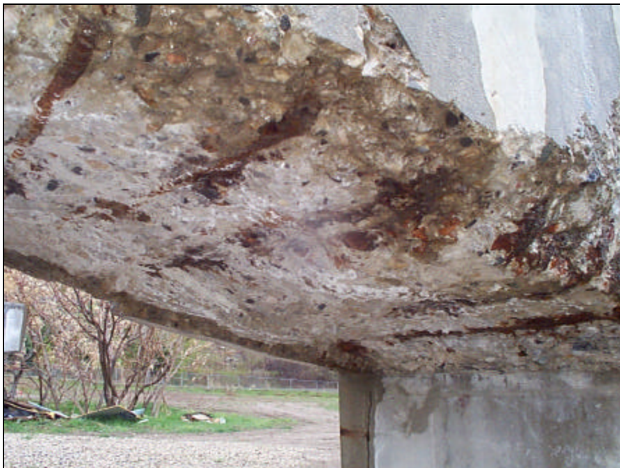
Figure 1.6 – Bent 12N, close up of deterioration on underside of cantilever
