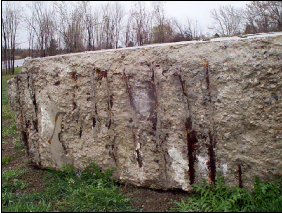
Figure 1.3 – Bent 12S, deterioration on underside of cantilever
