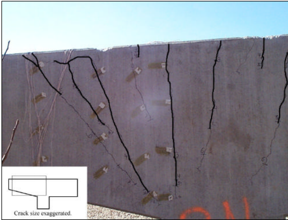
Figure 5.49 – Bent 2N, cracks on cycle 5.
