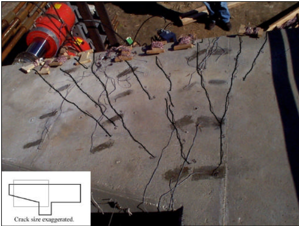
Figure 5.36 – Bent 1N, cracks on cycle 6.
