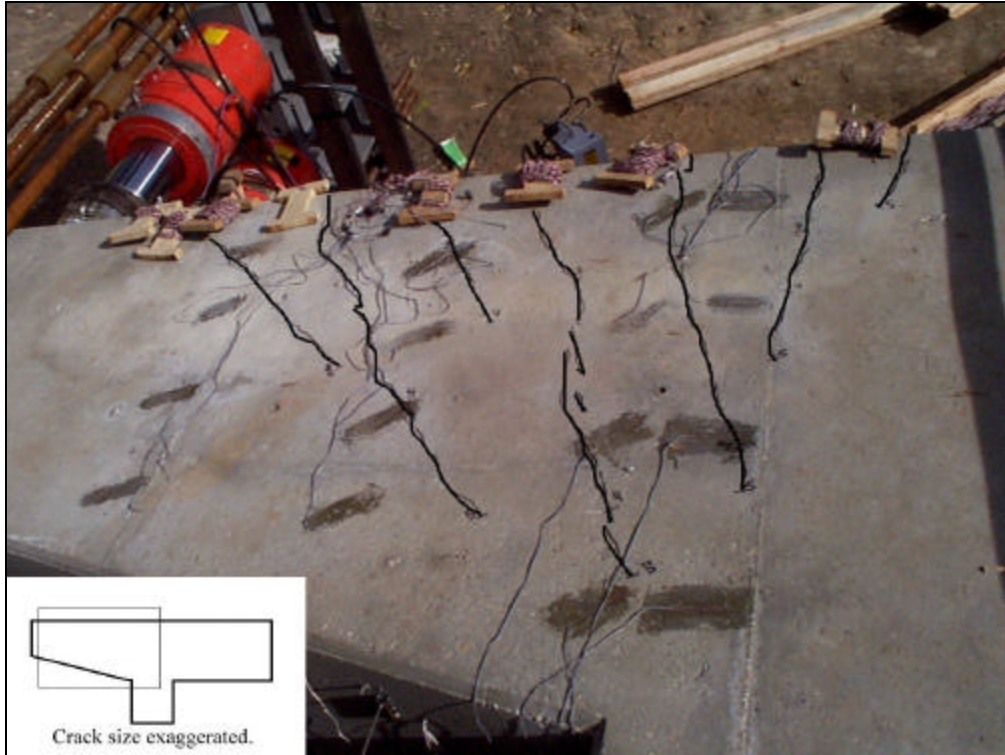
Figure 5.35 – Bent 1N, cracks on cycle 5.
