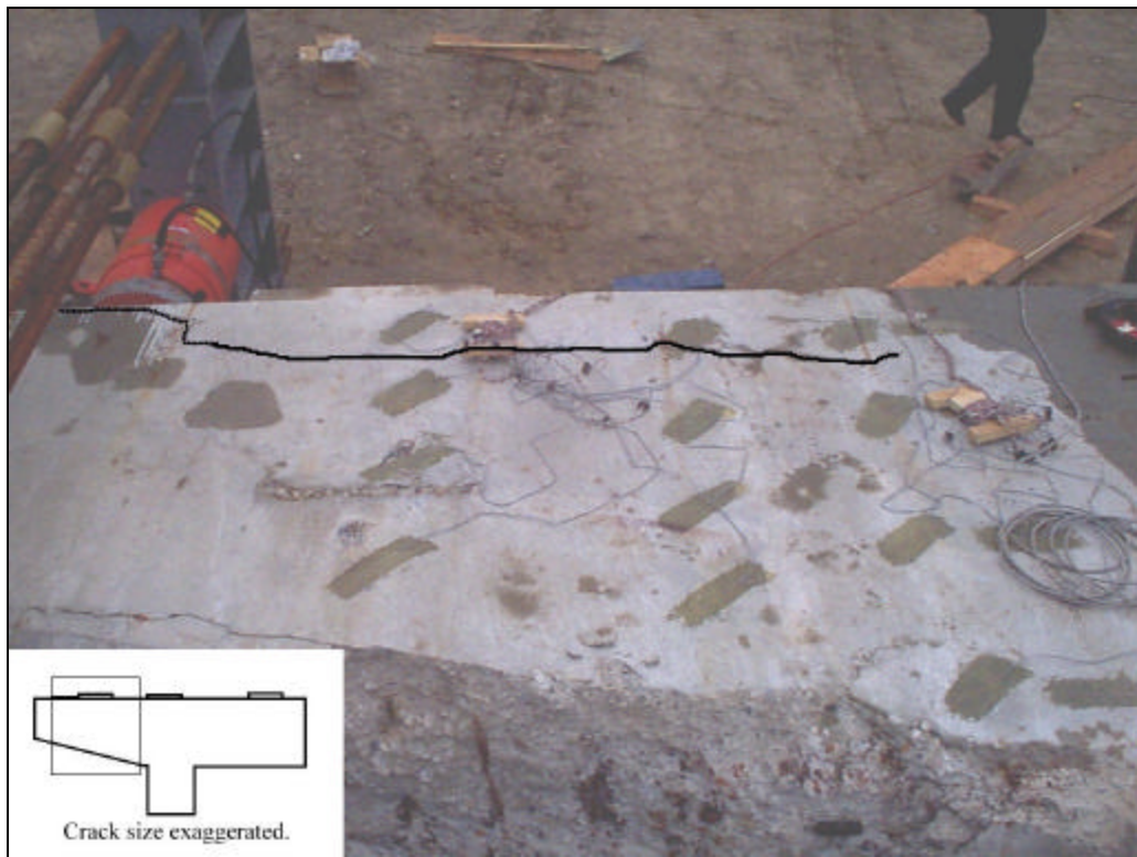
Figure 5.21 – Bent 12N, crack previous to testing, deterioration of underside of beam.
