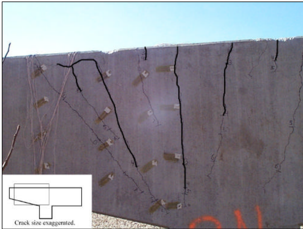
Figure 5.48 – Bent 2N, cracks on cycle 4.
