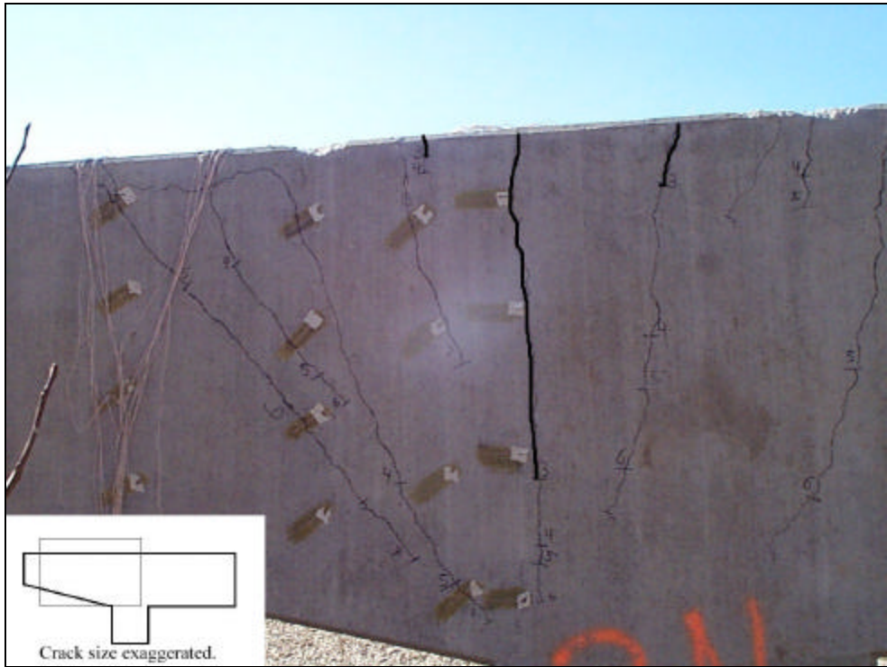
Figure 5.47 – Bent 2N, cracks on cycle 3.
