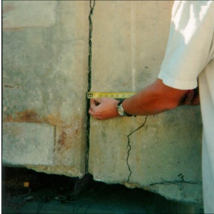
Figure 5.18 – Bent 12S, crack in reentrant corner of pedestal and top of bent.
