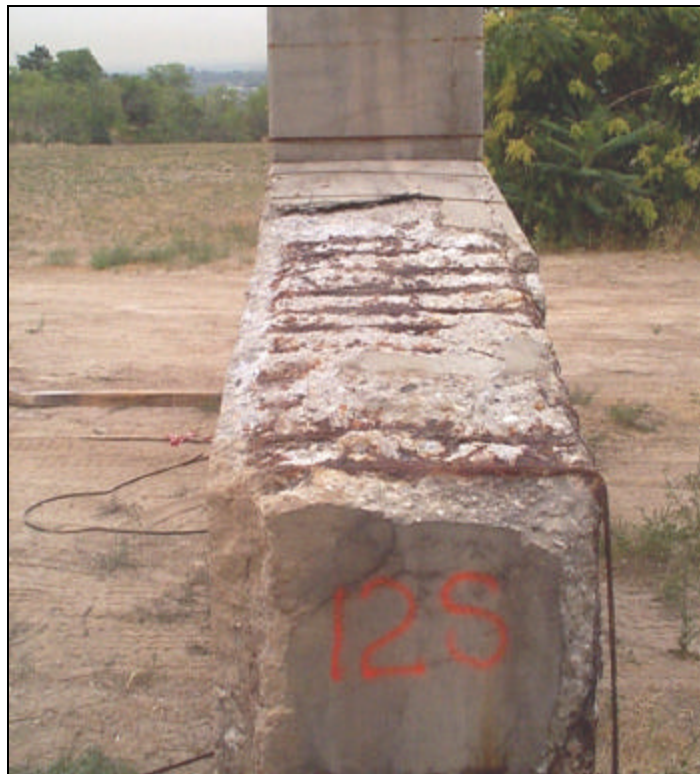
Figure 5.7 – Bent 12S, deterioration on underside of cantilever.
