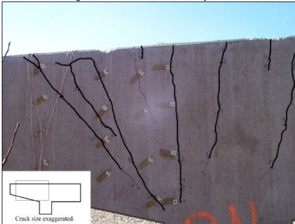
Figure 5.50 – Bent 2N, cracks on cycle 6.
