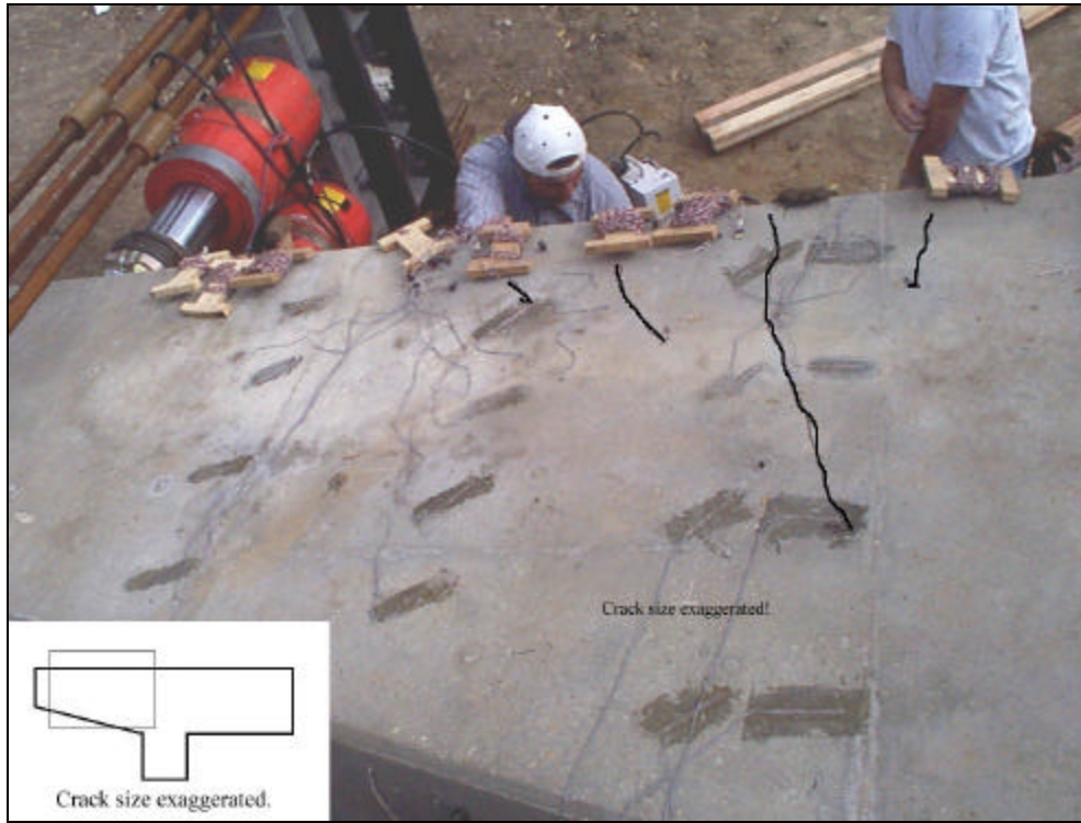
Figure 5.33 – Bent 1N, cracks on cycle 3.
