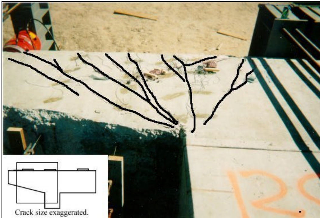
Figure 5.19 – Bent 12S, crack pattern at failure
