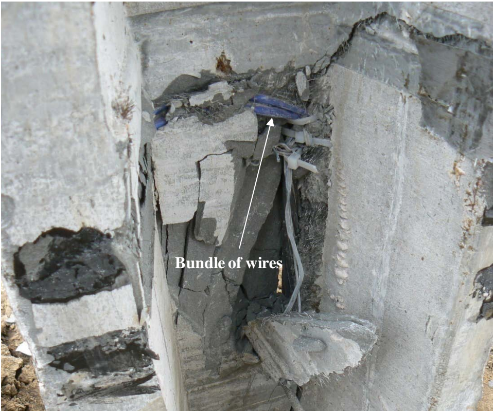
Figure 5.49. Shear failure region of UHPC pile P1 after the lateral load test with some cracked UHPC pieces removed
