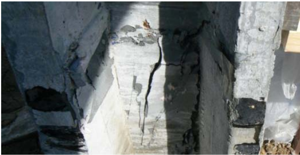
Figure 5.43. Initial shear cracking in web of UHPC pile P1 at a lateral load of 22.8 kip (101.3 kN)
