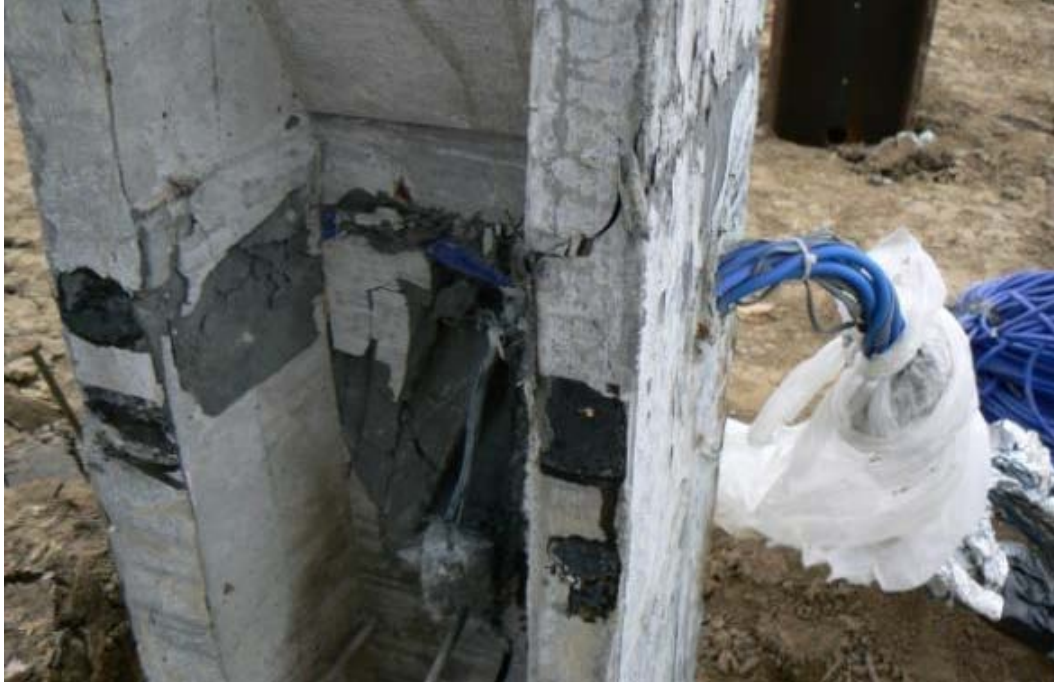
Figure 5.48. Bundle of instrumentation wires passing through the web and out of the flange of UHPC pile P1
