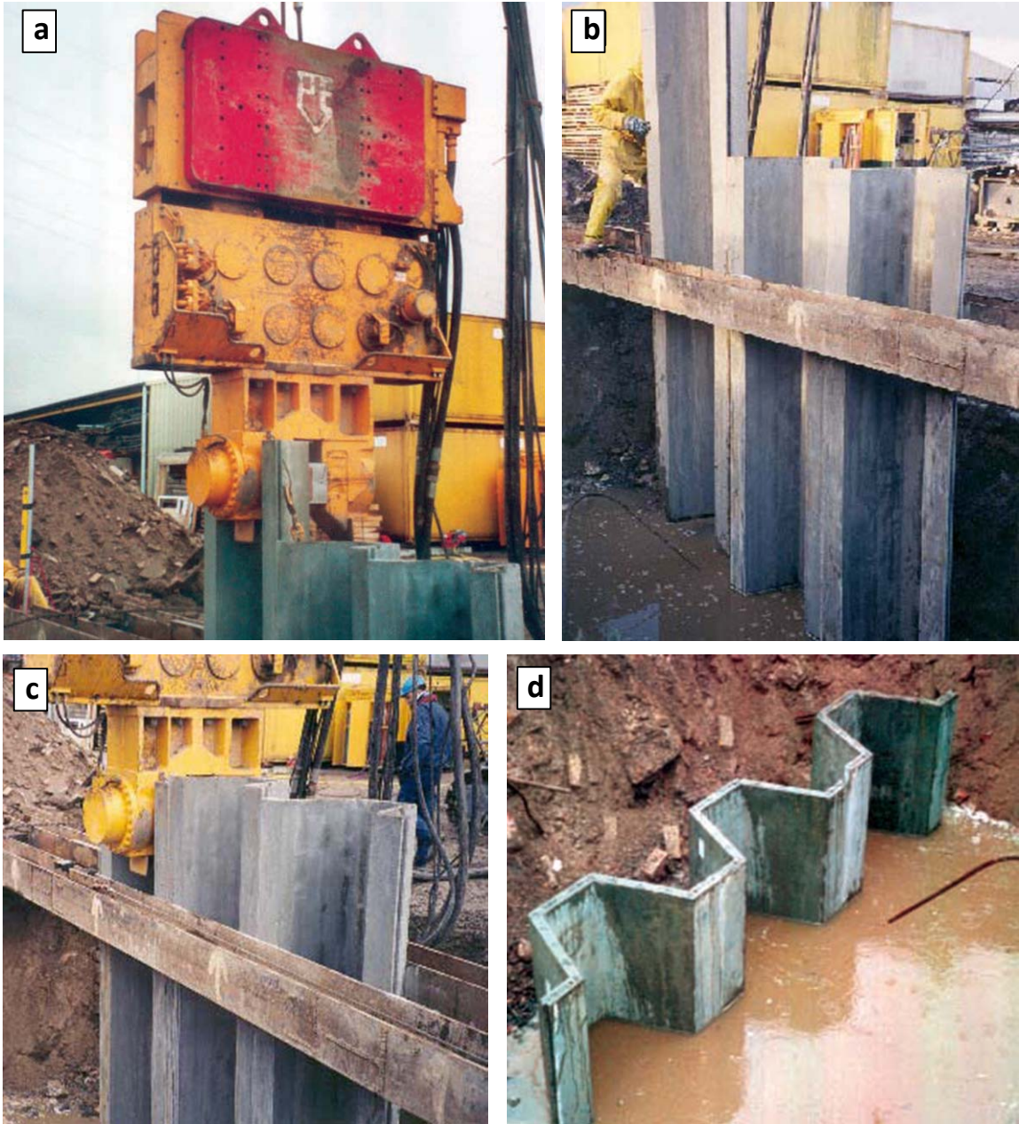
Figure 2.44. Views of a) to c) the driving process for SCFRC sheet piles and d) the completed view (Walraven 2007, Walraven and Schumacher 2005)
