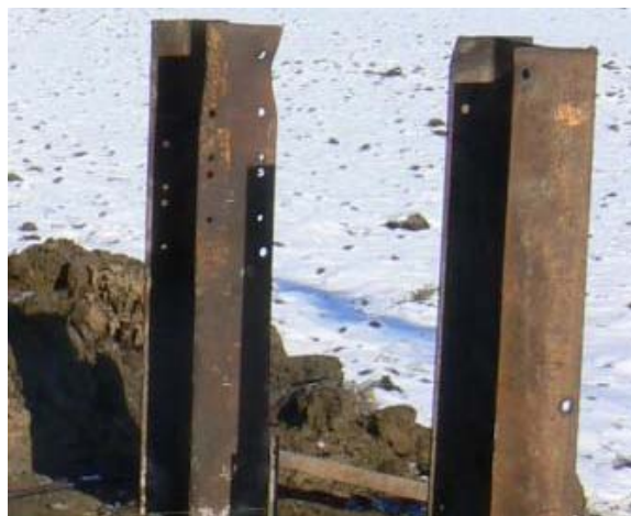
Figure 5.8. Local buckling and bending damage to two steel anchor piles due to driving
