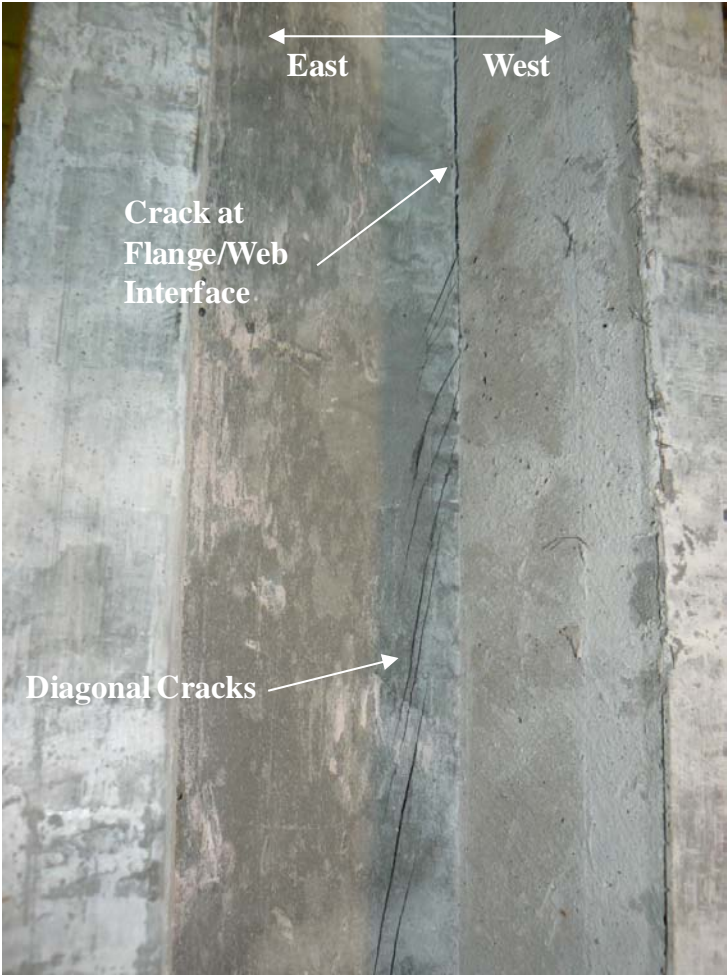
Figure 4.32. Diagonal cracking in test unit L2 at a lateral load of 5.2 kips (23 kN) (pull)
