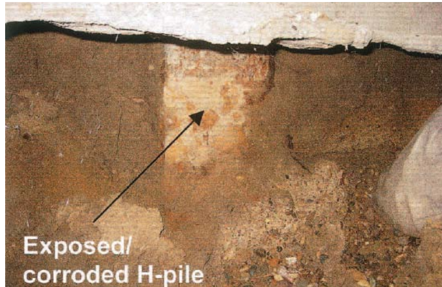
Figure 1.9. Corroded H-pile supporting integral abutment (White et al. 2007)
