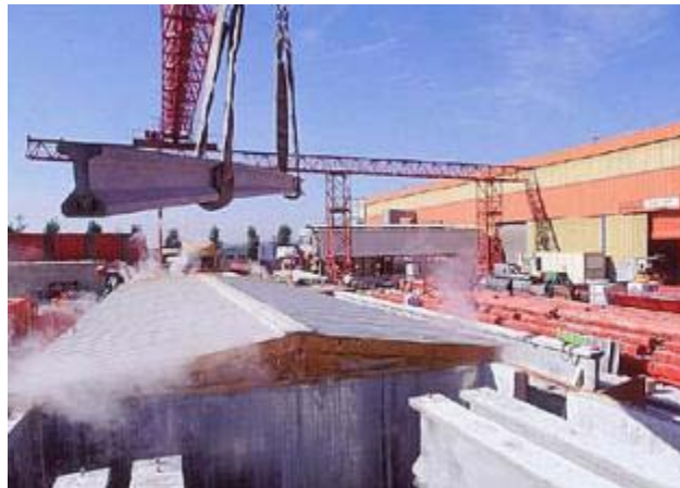
Figure 2.31. View of precasting area for UHPC beams for Cottenom Nuclear Power Plant (Lafarge North America 2007)
