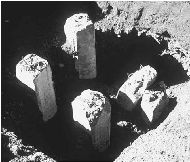
Figure 1.3. Damage to the tops of driven concrete piles due to unsuitable driving hammer size (Salgado 2006)
