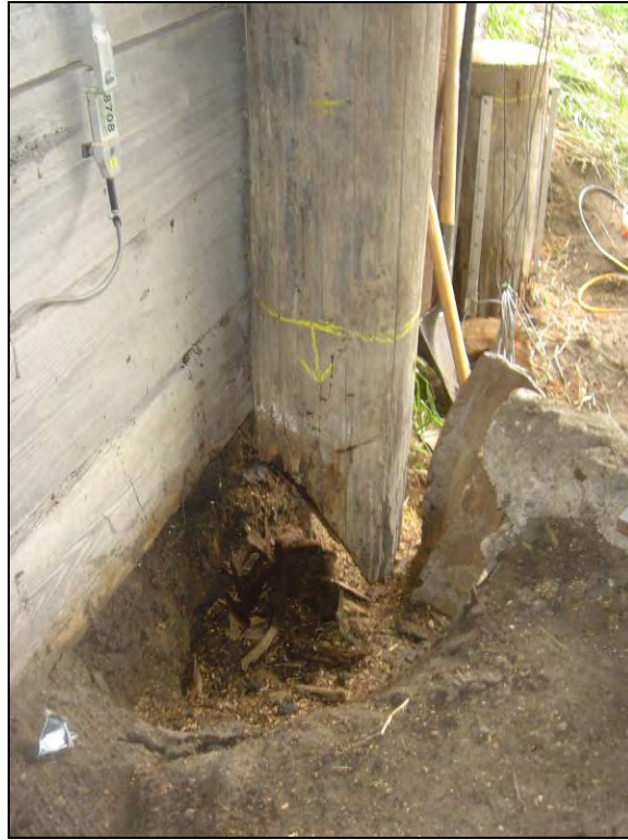
Figure 12.20. A section of Pile no. 6 removed near the ground level (Bridge No. 029070 Humboldt County – July 12 2006)
