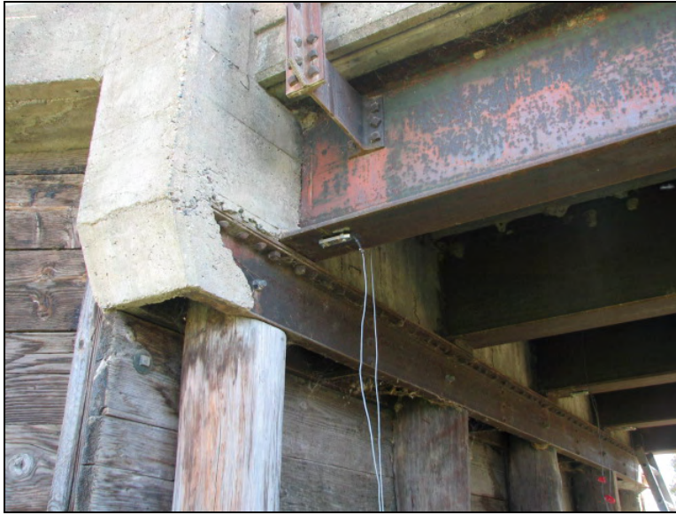
Figure 9.13. Pile cap partially resting on the timber backwall (Bridge No. 237350 Mahaska County – October 28 2005)
