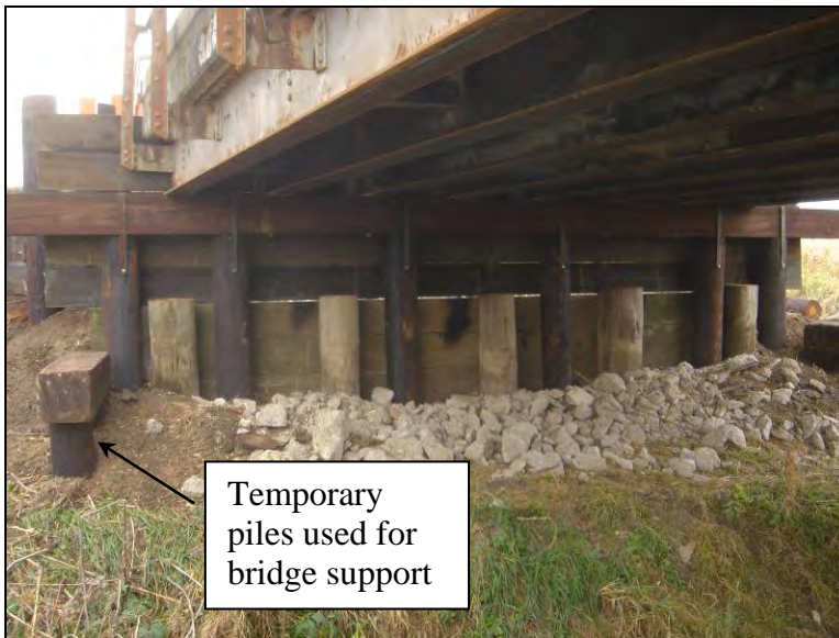
Figure 4.13. New timber abutment system constructed at the north side (Bridge No. 31-72-50 Tama County – September 8 2005)
