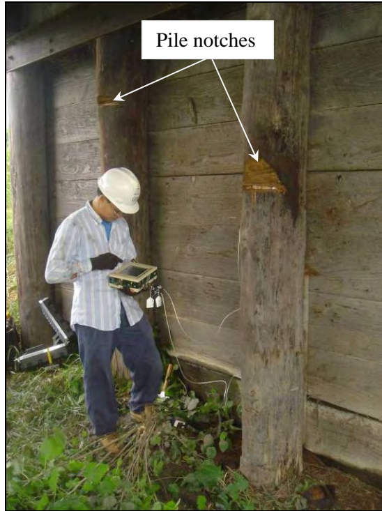
Figure 9.23. Notches created in the exposed piles to allow for axial impact (Bridge No. 237350 Mahaska County – August 17 2006)
