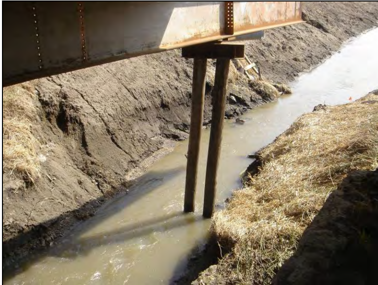
Figure 12.3. Center pier supported by 2 timber piles on each side of the bridge (Bridge No. 029070 Humboldt County – April 4 2006)
