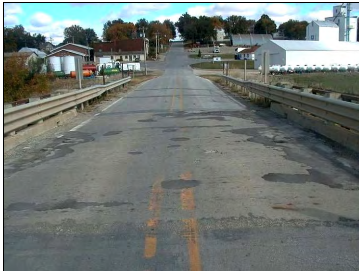
Figure 10.2. Concrete deck patched with asphalt (Bridge No. 094680 Carroll County – May 16 2006)
