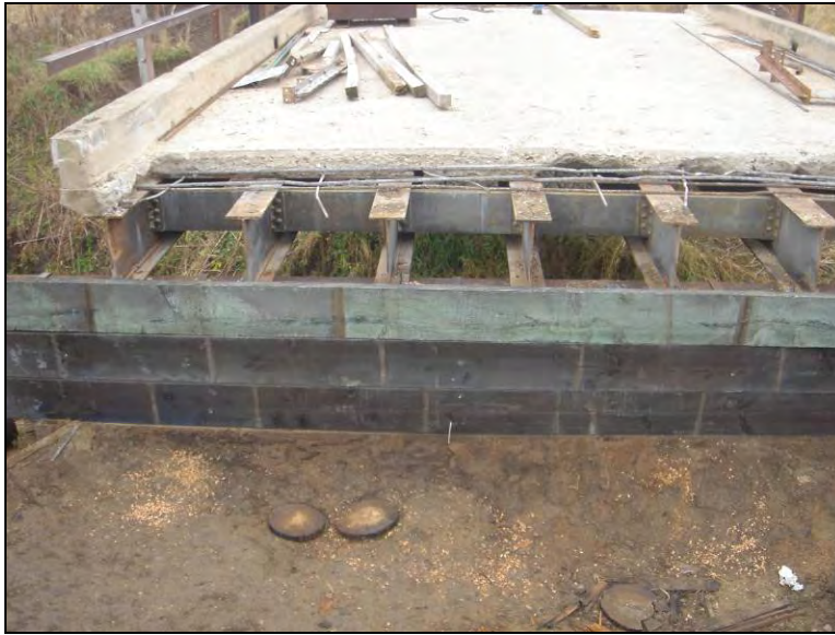
Figure 4.12. A section from the concrete deck is removed for driving timber piles (Bridge No. 31-72-50 Tama County – September 8 2005)
