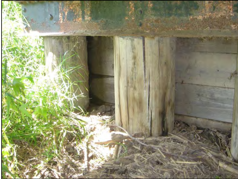
Figure 8.6. Hammer sounding and probing revealed a hollow core at pile no. 2 at the north abutment (Bridge No. 243470 Marshall County – June 22 2005)
