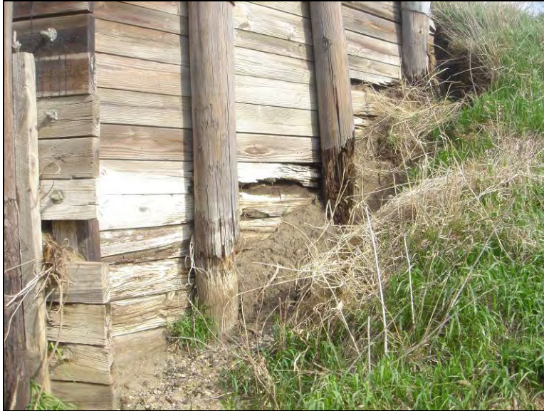
Figure 10.4. Severe deterioration observed at the northeast wingwall piles (Bridge No. 094680 Carroll County – April 15 2006)
