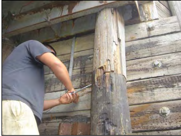
Figure 12.22. Metal screws used to connect the new section to the existing timber pile (Bridge No. 029070 Humboldt County – July 12 2006)
