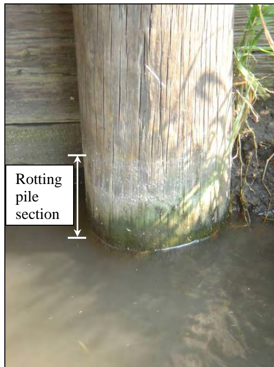
Figure 7.7. Soft section at pile No. 7 above the water level (Bridge No. 7710 Boone County – July 1 2005)
