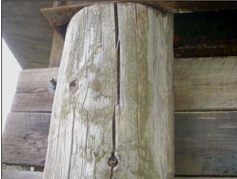
Figure 4.2. Pile cracking near the pile top (Bridge No. 1045 Black Hawk County – April 2 2005)
