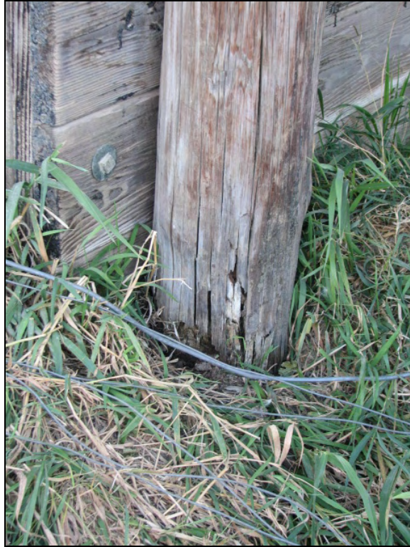
Figure 9.4. Biological deterioration of pile No. 1 at the ground level (Bridge No. 237350 Mahaska County – October 25 2005)
