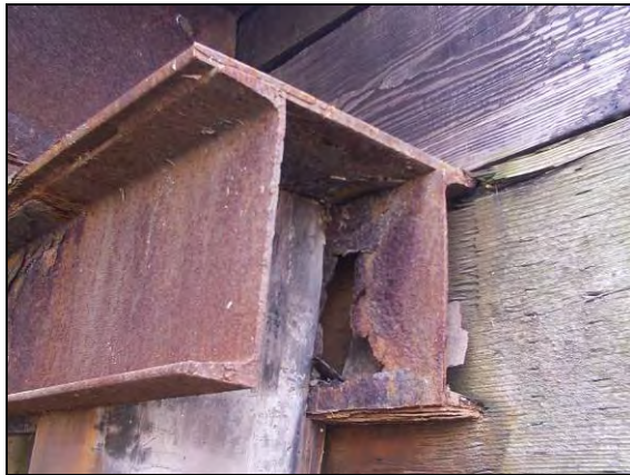
(a) Corroded steel (Bridge No. 1045 Black Hawk County – April 2 2005)
