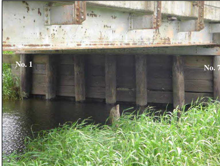
Figure 7.2. Seven supporting timber piles at each abutment with a timber backwall and double c-channel cap (Bridge No. 7710 Boone County – June 1 2005)
