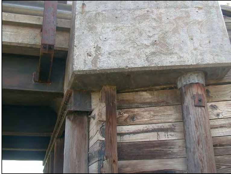
Figure 10.14. Pile cap partially resting on the backwall (Bridge No. 094680 Carroll County – May 16 2006)
