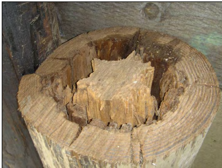
Figure 5.1. Significant internal pile deterioration that is difficult to detected using the stress wave technique (Bridge No. 31-72-50 Tama County – June 10 2005)
