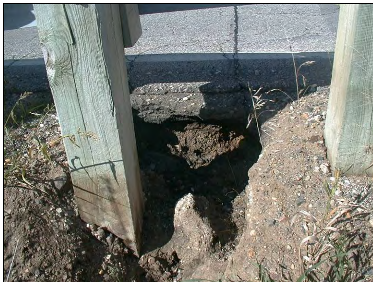
Figure 10.3. Soil erosion near the north abutment (Bridge No. 094680 Carroll County – April 15 2006)
