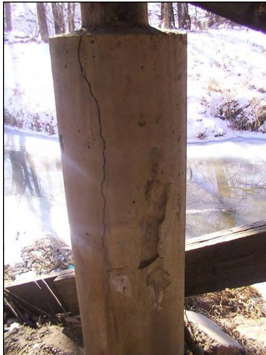
Figure 4.9. Spalling and cracking of concrete casing (Bridge No. 149 Boone County – February 11 2005)
