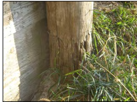
(b) Brooming of pile at the east end of the north abutment
