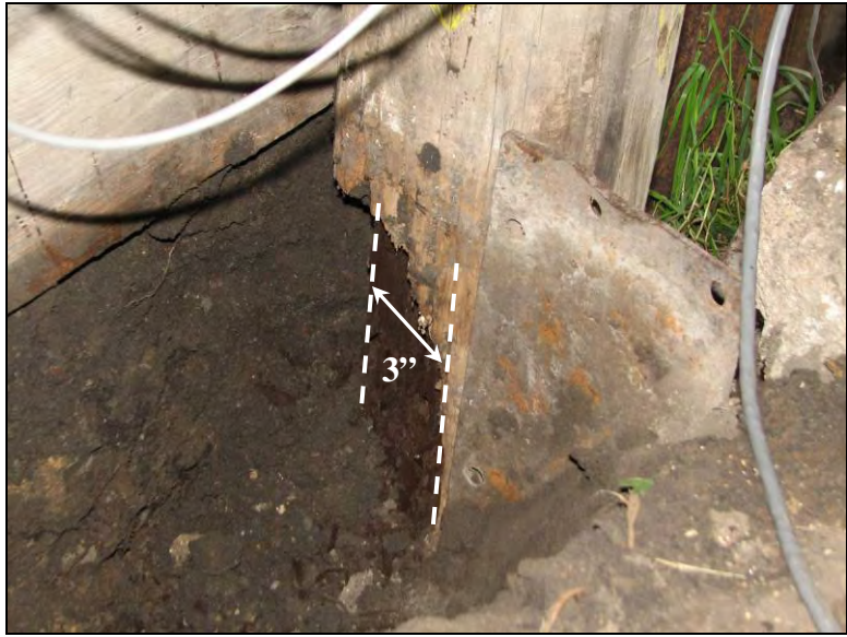
Figure 12.9. Advanced section loss at pile No. 6 at the east abutment (Bridge No. 029070 Humboldt County – July 12 2006)
