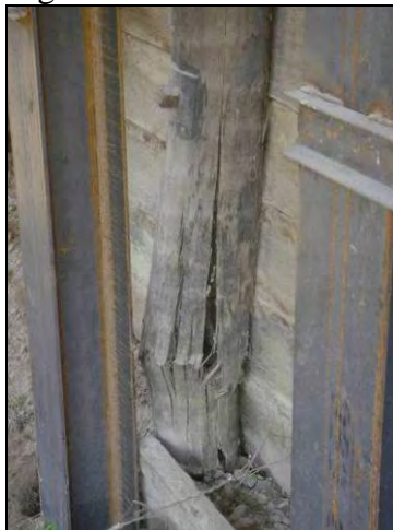
(c) “Mushrooming” of fibers at a hollow section (Bridge No. 23-70-00 Mahaska County – July 8 2005)
