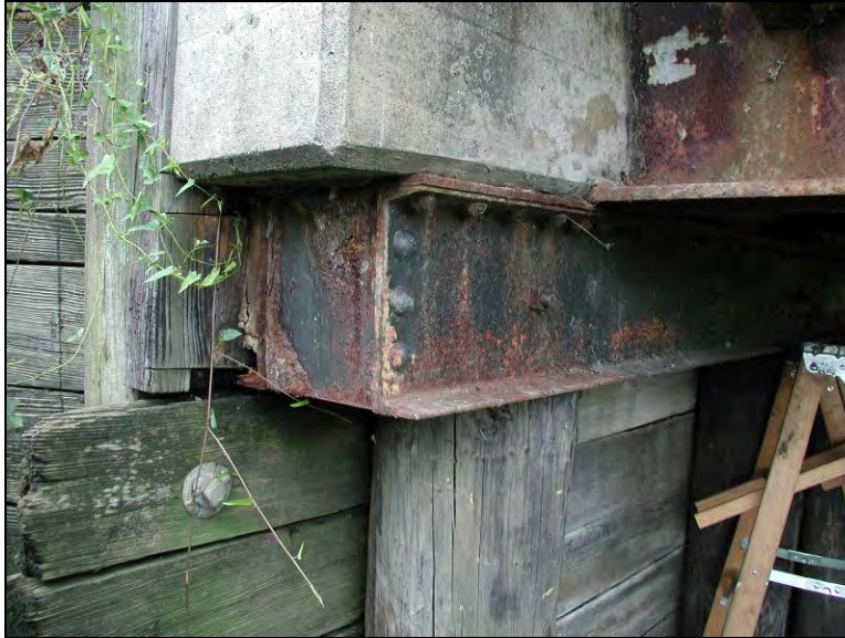
Figure 8.18. Pile cap partially resting on the timber backwall (Bridge No. 243470 – Marshall County – July 28 2005)
