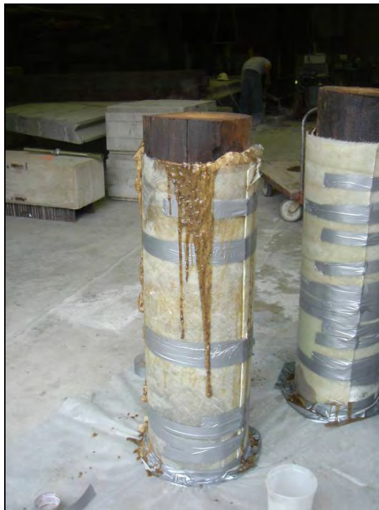
Figure 13.14. Expandable wood filler epoxy applied to fill the void between the pile and the FRP shell
