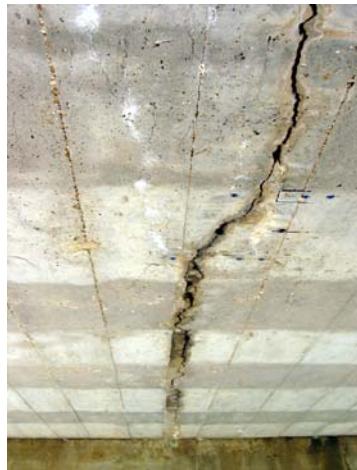
Figure 1-3 - Soffit Slab Longitudinal Crack
