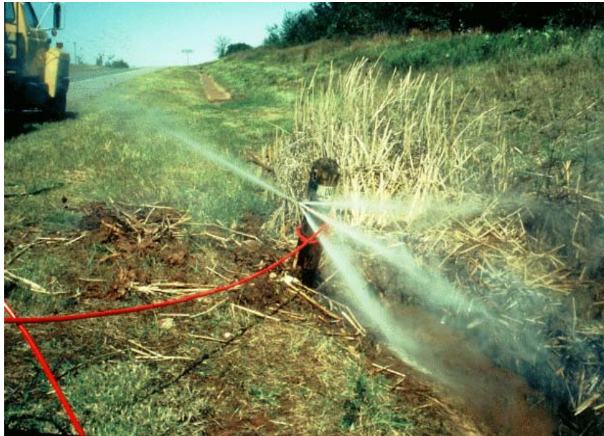
Figure 6.10. Pipe flushing unit (Baumgardner, 2002).
