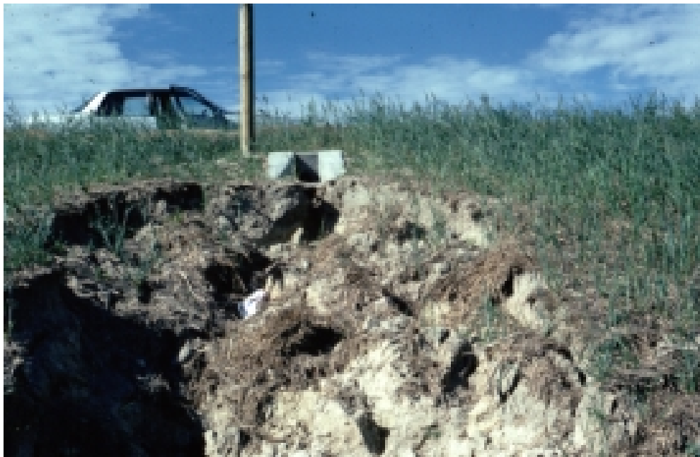
Figure 6.7. Excessive erosion at the outlet pipe (Baumgardner, 2002).
