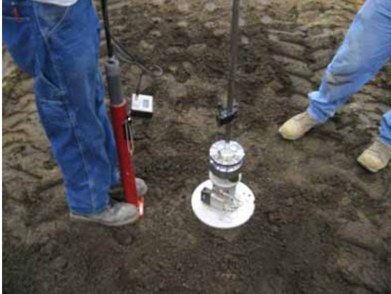
Figure 8. Strength and stiffness determination using Clegg impact hammer (left) and PFWD (right)
