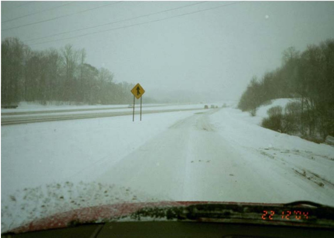
Figure 16 : Picture documenting typical road condition on freeway entrance ramp to I-271 on December 22, 2004. The road is covered with snow.
