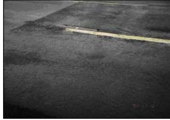
b) Low Quality Transverse Joint
