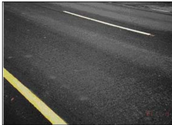
Figure 16: Wash Boarding Effect
