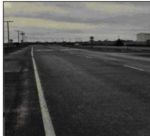
b) Poor Quality Longitudinal Joints
