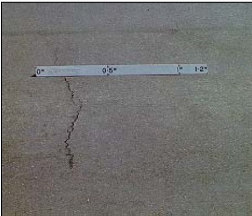
(Direction of Travel →) Figure 3: Transverse Cracking
