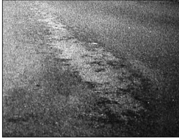
Figure 17: Traffic Damage Caused by Early Trafficking
