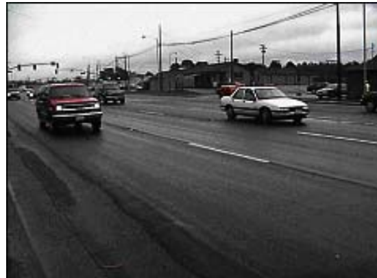
b) Poor Quality Edges and Shoulder
