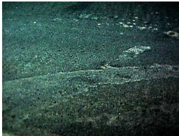
Figure 18: Damage Due to Post Application Heavy Rain with Shear
