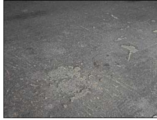
b) Delamination from a False Slurry
