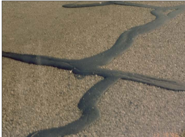
Figure 25: Poor Workmanship – Raised, Bumpy Sealing
