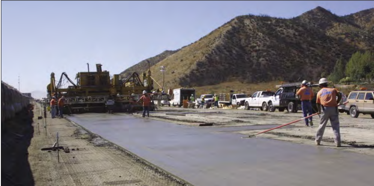
Crews constructing a special lane for large trucks on the I-5 Devore project
