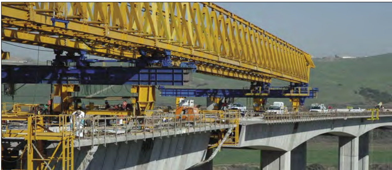
The last pre-cast segment of new SR-125 is placed for the Otay River Bridge, the first toll road in San Diego County.
