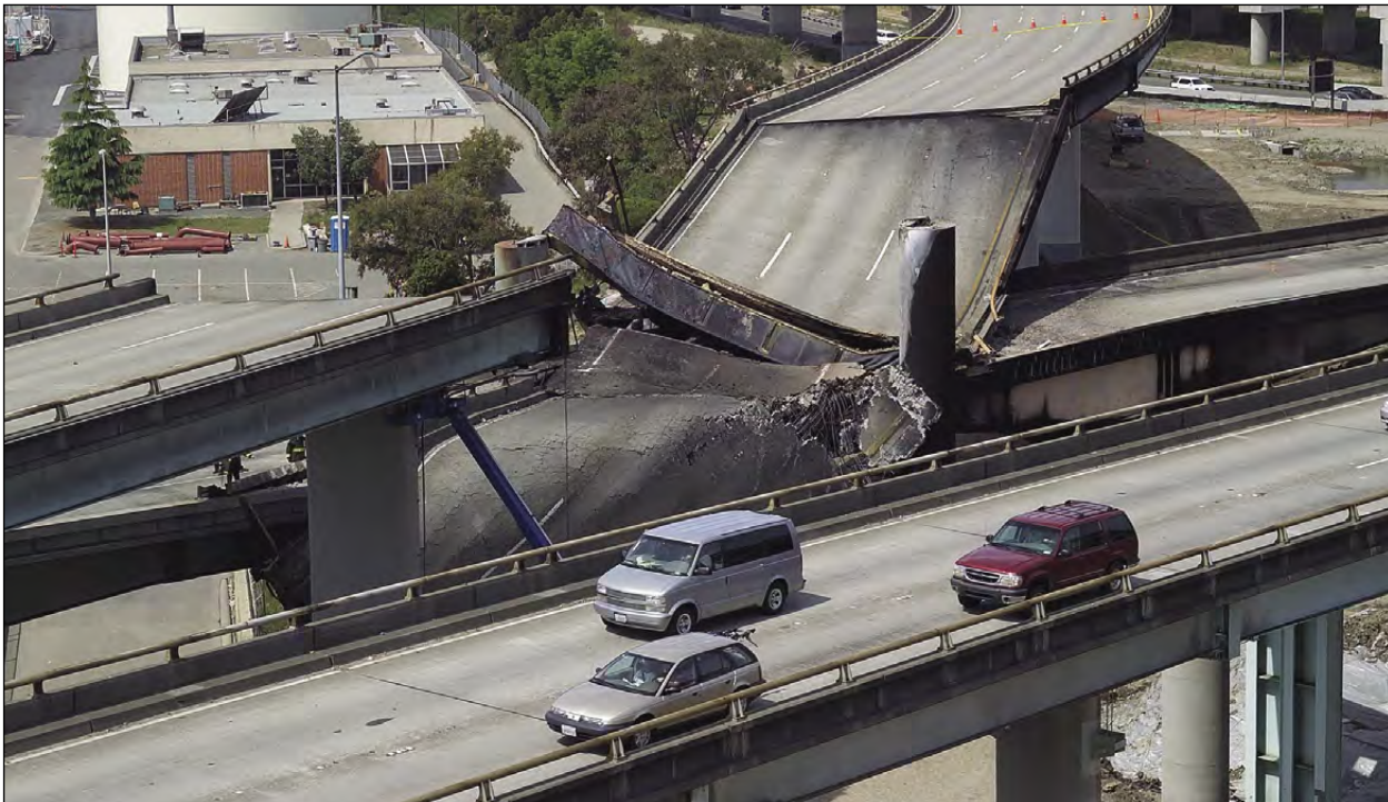
Damaged I-580 connector that fell onto I-880 section of Oakland's MacArthur Maze
