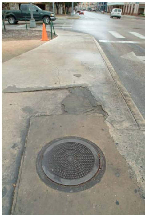
Figure 7-14. Utility Cover in the Pedestrian Path at Southeast Corner.
