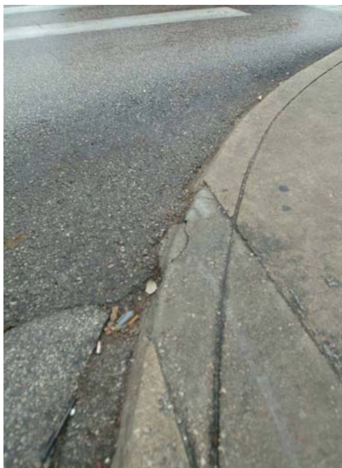
Figure 7-16. Uneven Pavement and Change in Level at Southeast Corner of Intersection.
