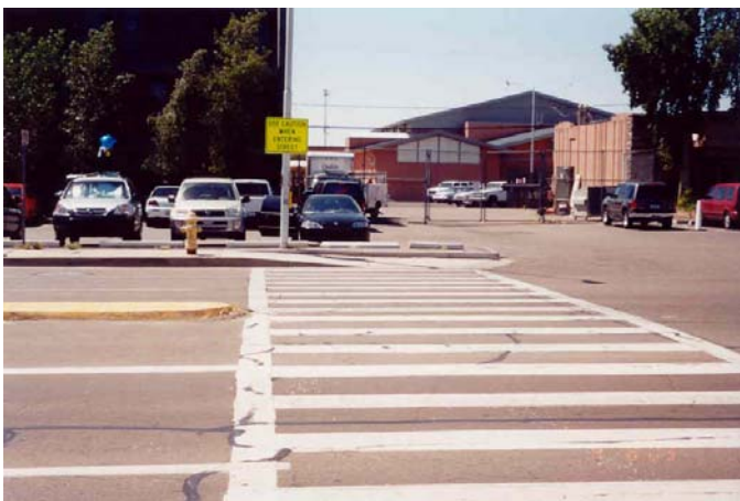
Figure 7-21. Example of High-Visibility Markings.
