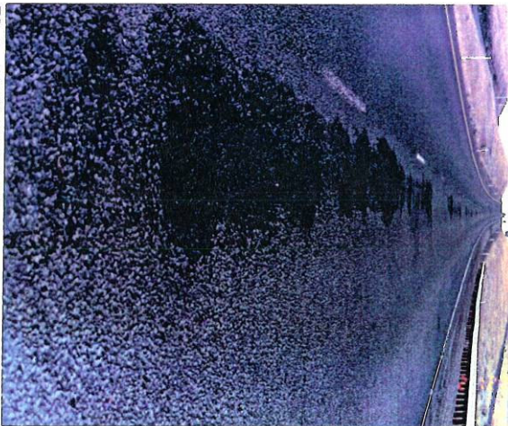
Photo 6, MP 207.91, Westbound Truck Lane Potholes that have required maintenance patching.
