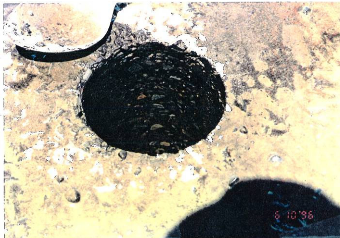
Photo 14, MP 205.73, Westbound Truck Lane Core taken in the center of lane. The underlying Asphalt Class B looks good.
