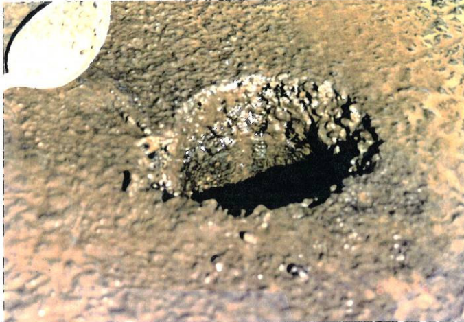
Photo 23, MP 194.88, Eastbound Truck Lane Stripping occurring within the top 0.25 to 0.30 ft of MCD and Class D.
