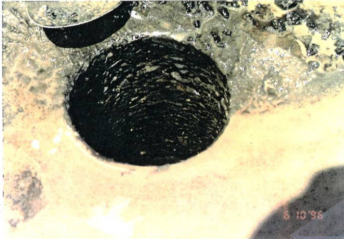
Photo 9, MP 205.73, Westbound Truck Lane Stripped Asphalt Class B beneath the MCD surface in the left wheelpath. The MCD surface appears fat and the core appears very dense.
