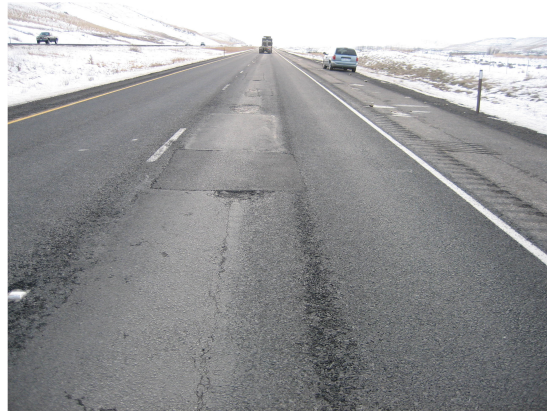
Figure 10. String of patches typical to distressed areas.
