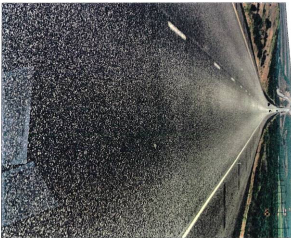
Photo 18, MP 195.00, Eastbound Truck Lane Flushing appearing in the eastbound truck lane.
