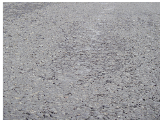
Figure 8. Area with fat spots beginning to crack.
