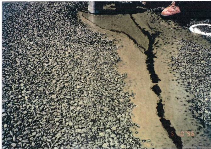
Photo 2, MP 202.49, Westbound Truck Lane Left wheel path where the MCD surface has become fat.
