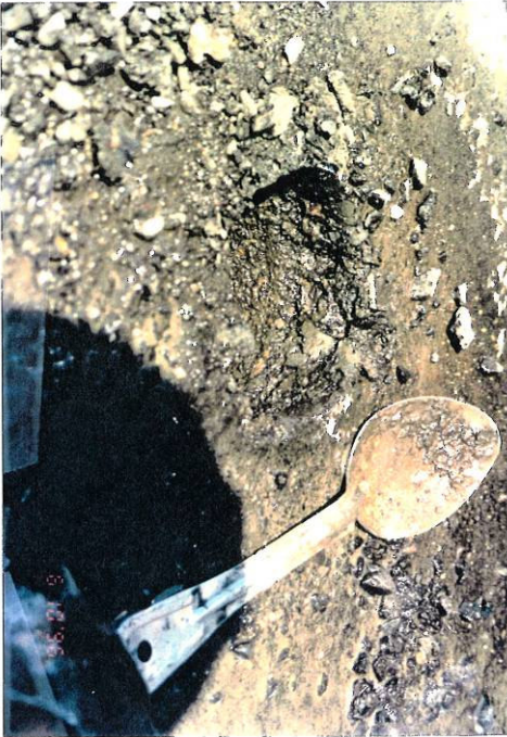
Photo 11, MP 206.62, Westbound Truck Lane Stripped Asphalt Class B beneath the MCD surface in the left wheelpath. The MCD surface appears fat and the core appears very dense.
