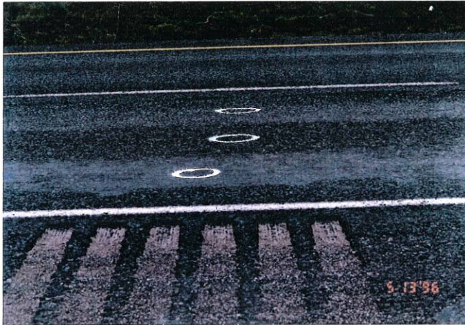
Photo 3, MP 208.01, Westbound Lanes Wheelpaths in the truck lane where the MCD has turned fat.
