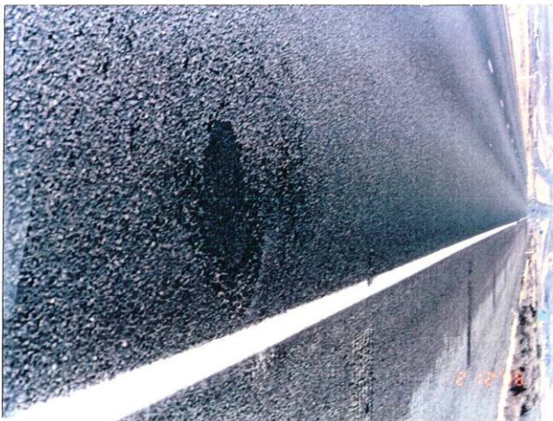
Photo 20, MP 195.75, Eastbound Truck Lane Isolated pothole. Stripping occurs almost full thickness.
