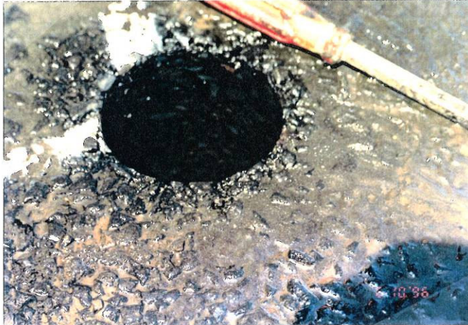
Photo 13, MP 202.37, Westbound Truck Lane Core taken in the center of lane. The underlying asphalt Class B looks good.
