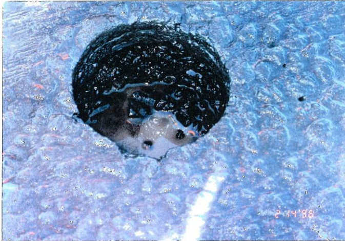
Photo 7, MP 207.87, Westbound Truck Lane Stripped Asphalt Class B beneath the MCD surface in the left wheelpath. The MCD surface appears fat and the core appears very dense.
