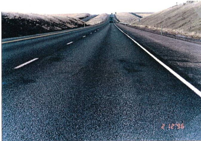
Photo 1, MP 208.09, Westbound Lanes Failing Modified Class D (MCD) surface. The wheel paths first appear fat, second push and shove, and finally potholes develop. This location shows several areas have almost progressed to potholes.
