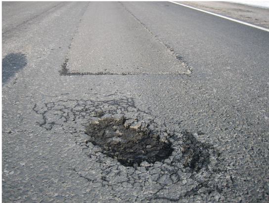
Figure 9. New pothole developing ahead of a previously patched area.
