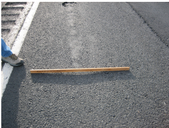
Figure 7. Fat spots and rutting in wheel path resulting from stripping.
