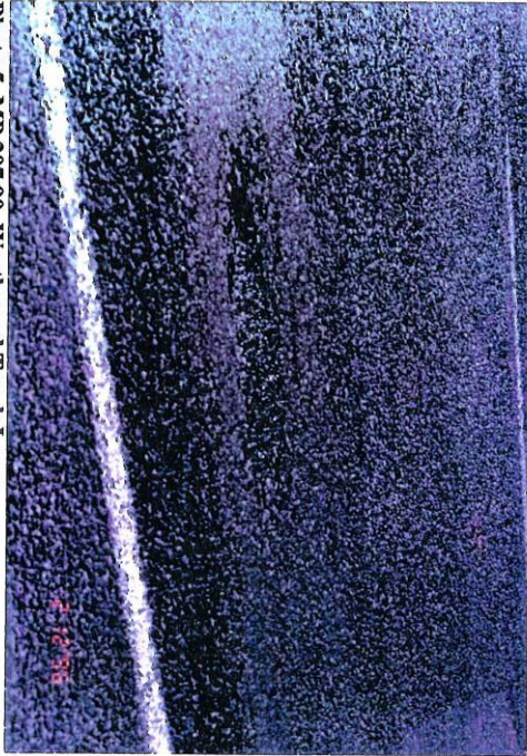
Photo 5, MP 207.90, Westbound Truck Lane Typical infancy stage of potholing of the MCD surface.
