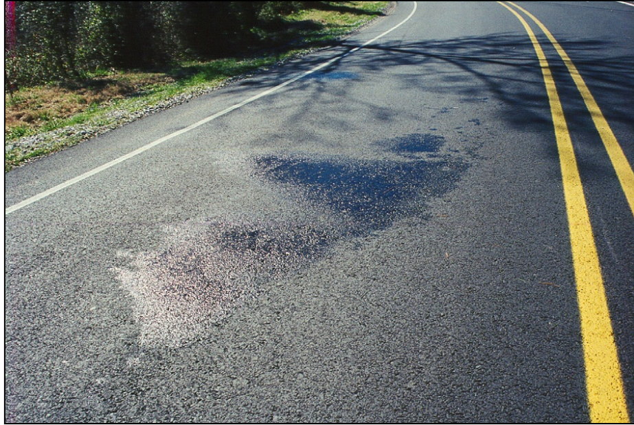
Figure 1. Pavement Structure “Weeping” Moisture
