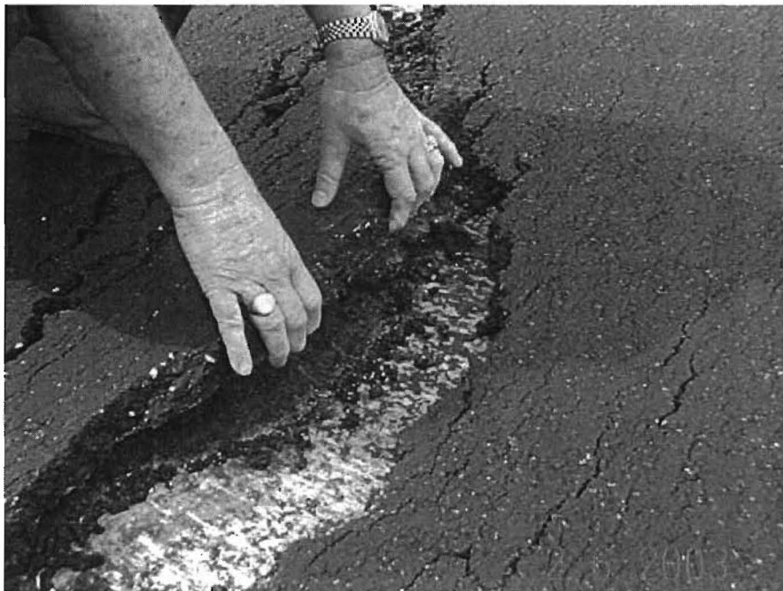
Figure 2.1 - Separation of Overlay Layer Due to Poor Bonding on US-17 in Florida
