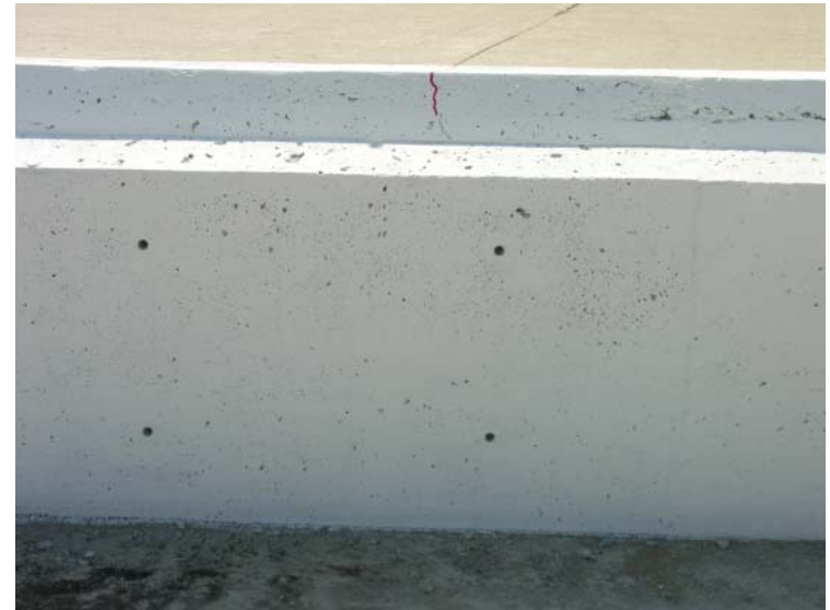
Figure 75. Barrier Cracks 4.6 m (15 ft) from Upstream End, Test TL5CMB-2
