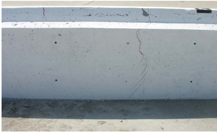
Figure 74. Barrier Cracks Upstream of Impact, Test TL5CMB-2
