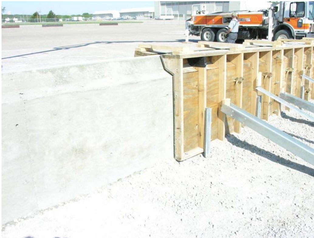
Figure 59. TL-5 Median Barrier Construction – Cold Joint
