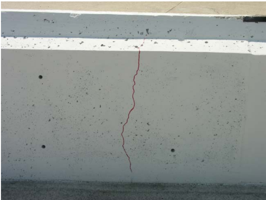
Figure 78. Barrier Cracks 12.2 m (40 ft) from Upstream End, Test TL5CMB-2
