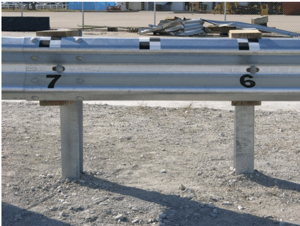
Figure 108. Post Nos. 5 through 7 Damage, Test MWT-5
