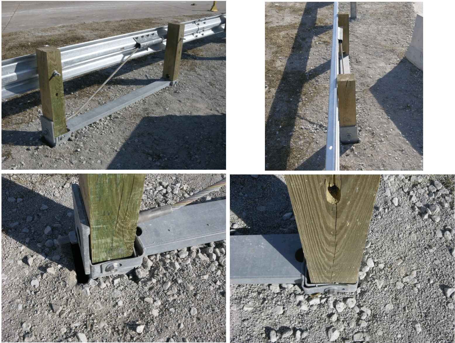
Figure 107. Anchorage System Damage, Test MWT-5
