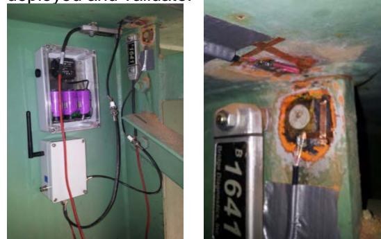
Wireless AE Sensor (Left) and Crack (Right)
