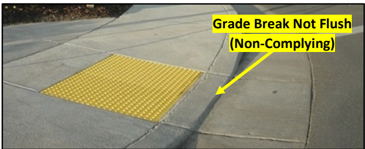
Figure 36: Non-Complying Grade Breaks
