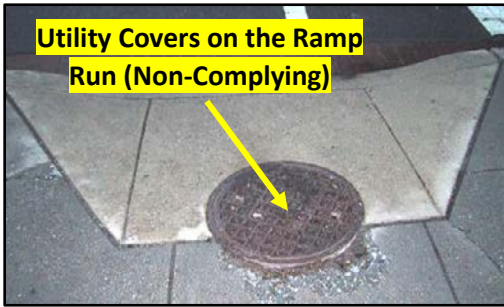
Figure 39: Non-Complying Utility Covers
