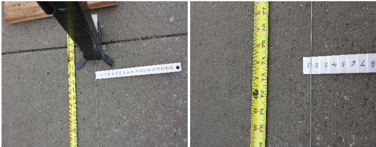
Figure 31. Profile measurements: at the joint (left) and at the center (right)
