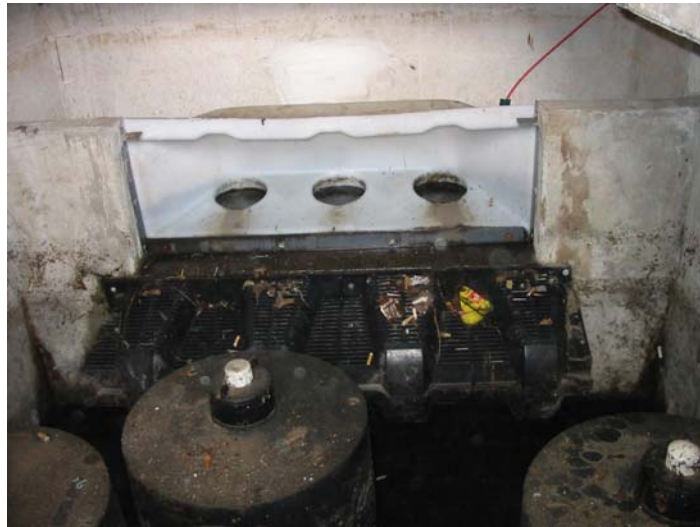
Figure 23. Cleanout of the settling bay and cartridge chamber for the stormwater filtration device. (Photo shows sediment and debris before cleanout.)
