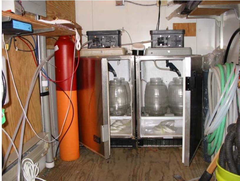
Figure 5. Automatic sampling equipment.
