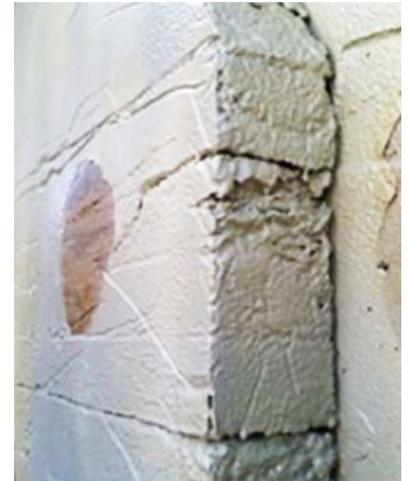
Serious cracking can be observed in this epoxy pourback, which encases a post tensioning anchorage (marked by the dark spot).
