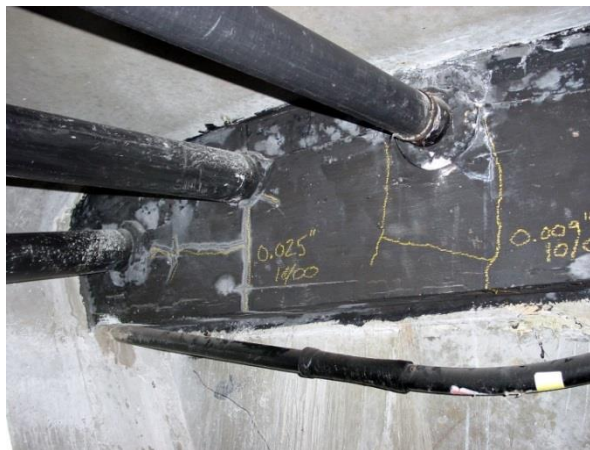
Figure 1-2: Pourback cracking on the Sunshine Skyway Bridge
