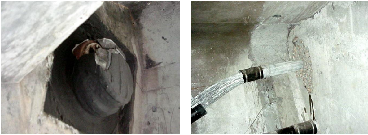
Figure 1-1: Tendon failure on the Mid-Bay Bridge
