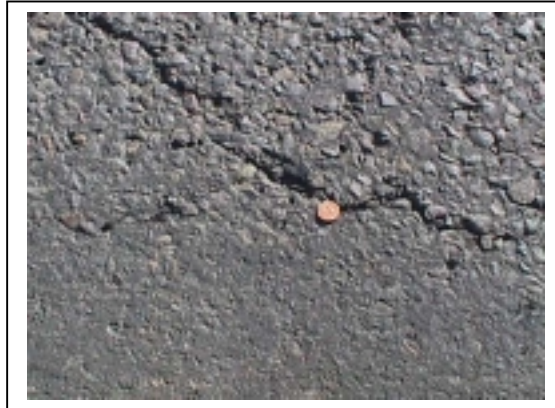
#29 Crack near 12.9 SB.
