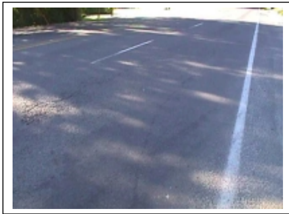
#26 looking south at D&S Harley Davidson – ravel and crack
