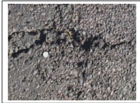
#33 Close-up of cracks near Compass Rose Store
