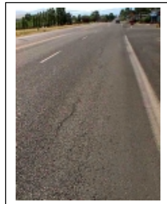
#35 Cracks in front of VRB Bank
