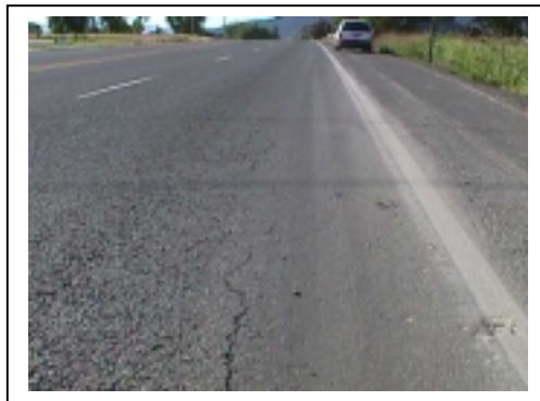
#30 Crack near 12.9 SB.
