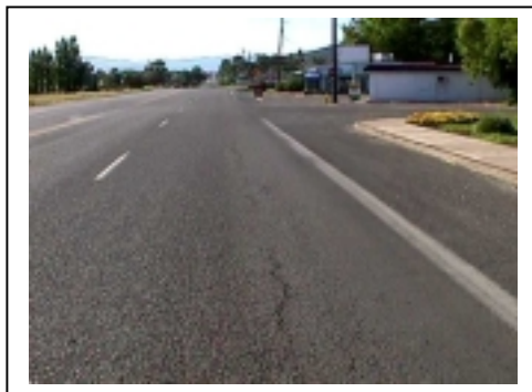
#34 Cracks in front of VRB Bank
