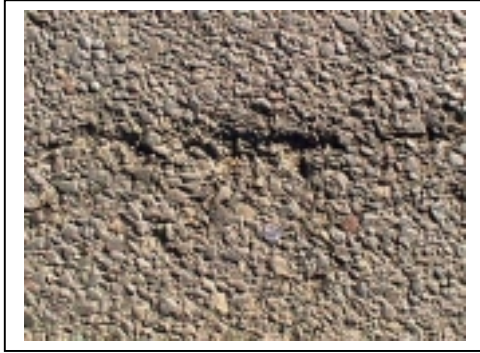
#3 Close-up of crack in front of Valley Forge Welding.
