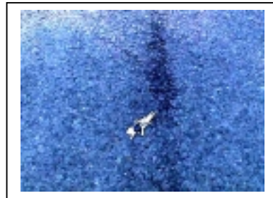
#18 Raveled area with crack.
