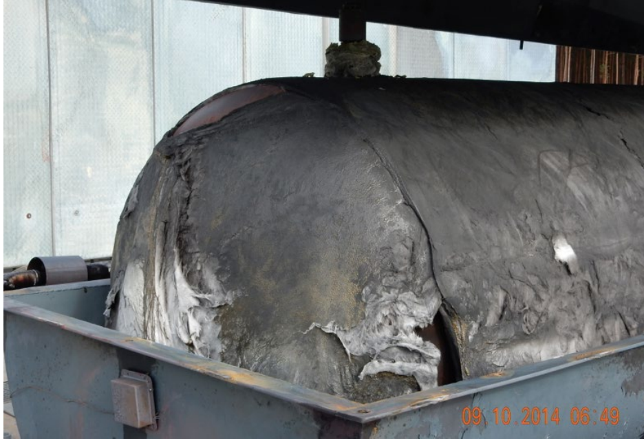
Figure 61. Test 2 - Insulation After Test
