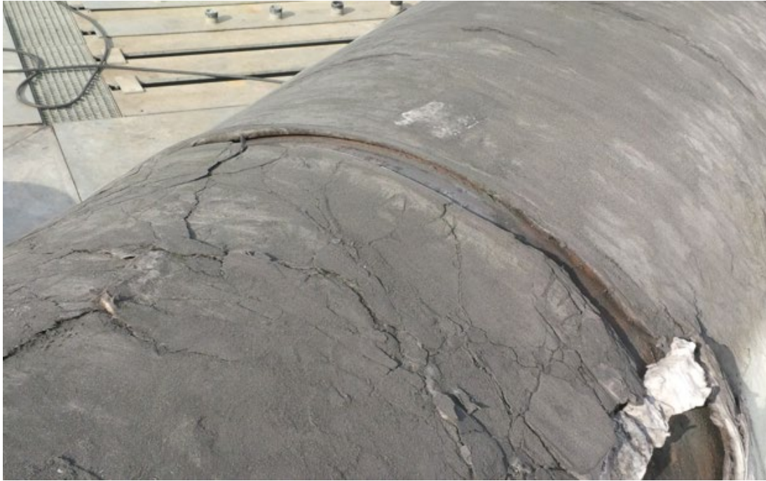
Figure 15. Test 1 - View of Separated Insulation on Tank Top at Mid Span. Picture also shows severe thinning of insulation.
