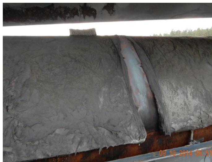
Figure 17. Test 2 - Insulation Separation at Mid-Tank
