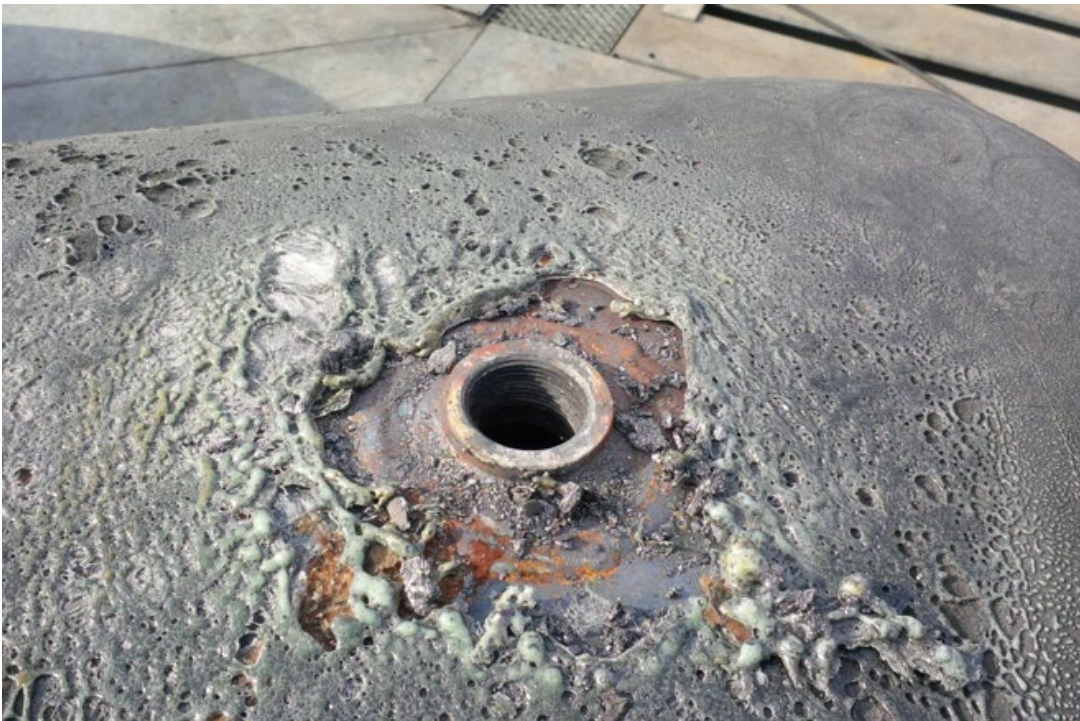
Figure 46. Test 1 - Burned Away Insulation at A-End Fill Fitting
