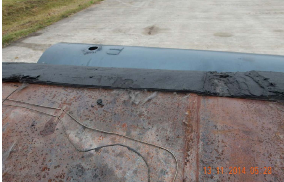
Figure 82. Test 4 - View of Insulation Thinning and Compaction
