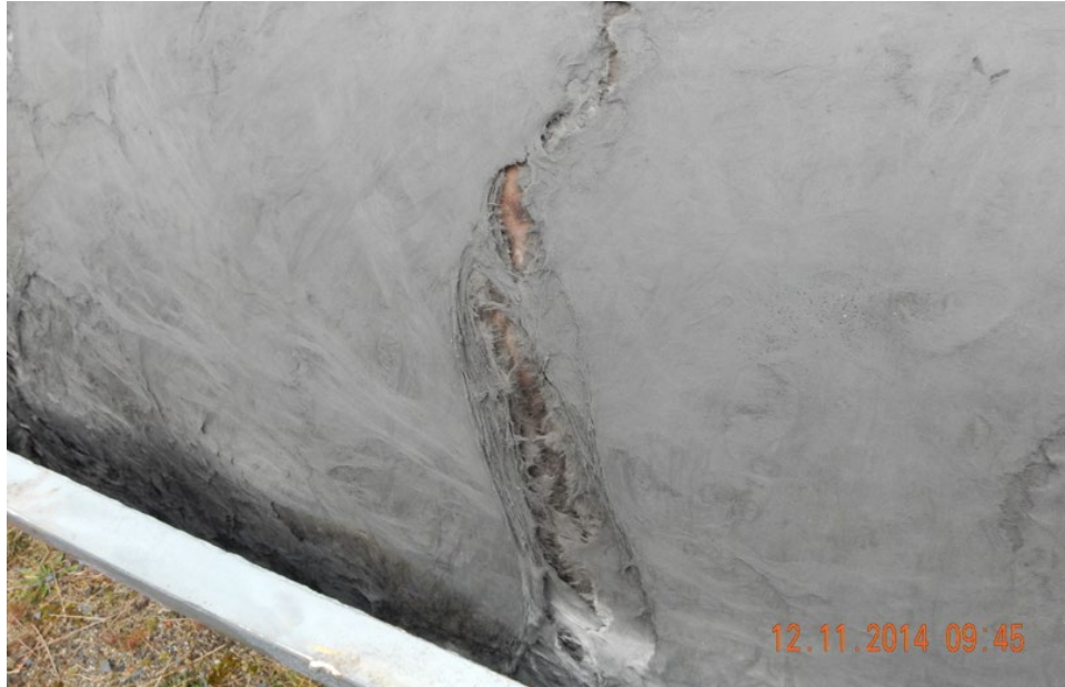
Figure 80. Test 4 - Insulation Stretch and Tearing on Tank Side
