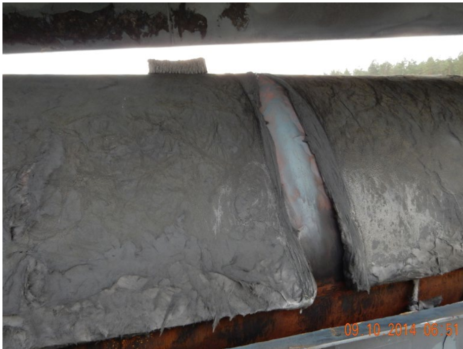
Figure 62. Test 2 - Insulation Gap at Mid Tank
