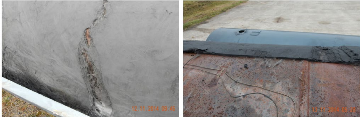
Figure 29. Test 4 – Images of Insulation Failure
