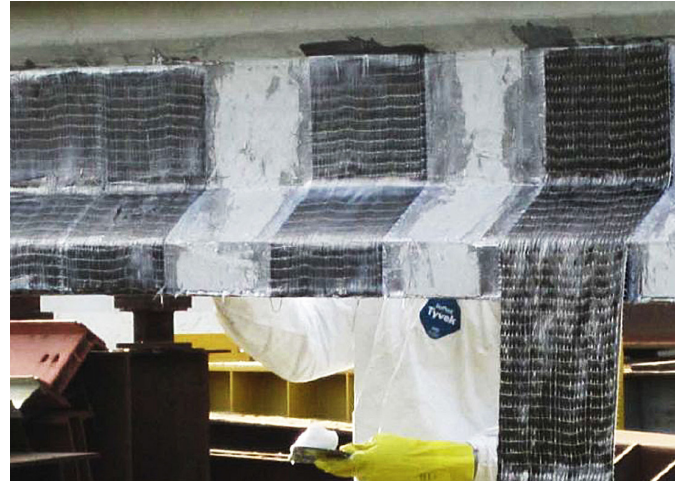
A technician works on wet layup application of CFRP fabric laminate on a prestressed concrete girder.
