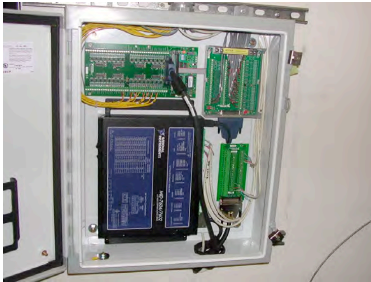
Figure 11. Main panel for data acquisition and control equipment. Top left AMUX-64T, top right SCB-68, bottom left MID-7604, bottom right CB68-LPR
