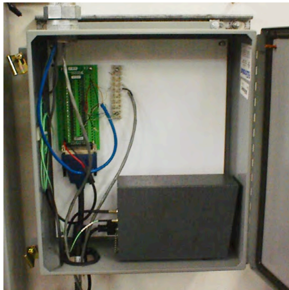
Figure 13. Control cabinet for cylinder pressure monitoring system
