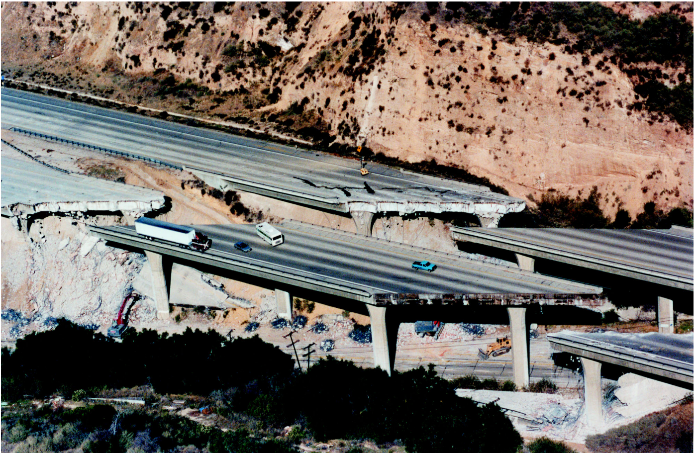
Figure 4. I-5 Damage at Gavin Canyon
